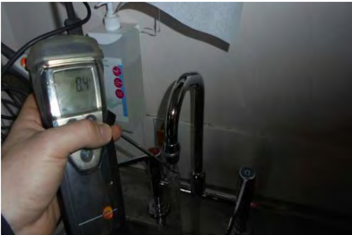
Treatment Room G/49 Sink – Cold Water Satisfactory After Extended Flush
