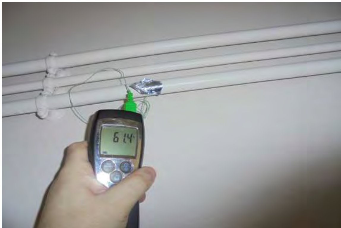
Health Education/Physio Room - Tertiary Loop Flow Temperature Satisfactory After Flushing Outlet
