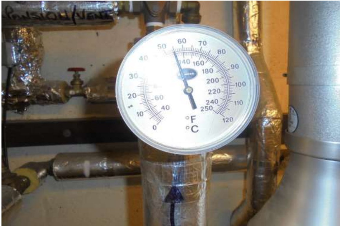
Gas Fired Water Heater No. 2 – Contents Temperature approx. 54°C
