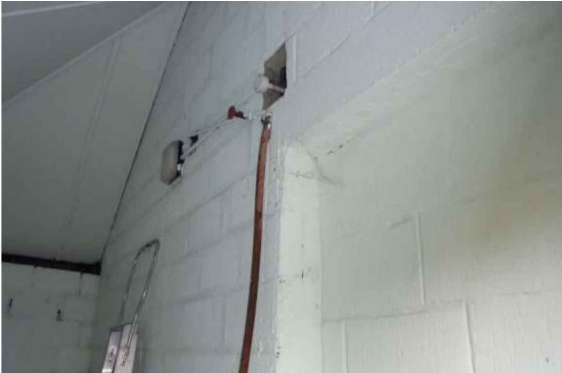
Bin Store MWS Connection – Effective Dead Leg
