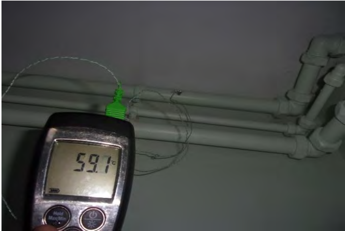
Secretarial Office (G/09) Hot Water Flow Temperature Satisfactory
