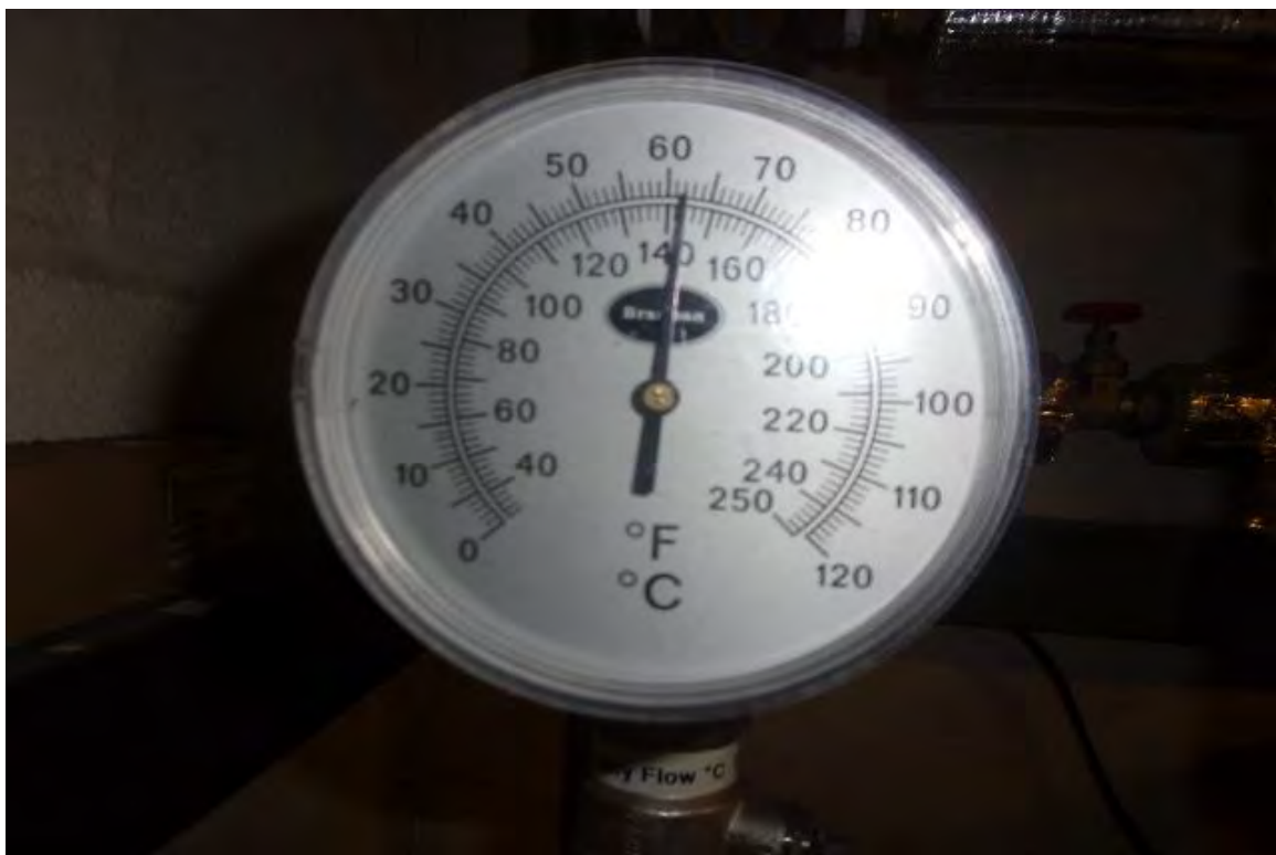
Gas Fired Water Heater No. 1– Contents Temperature approx. 62°C
