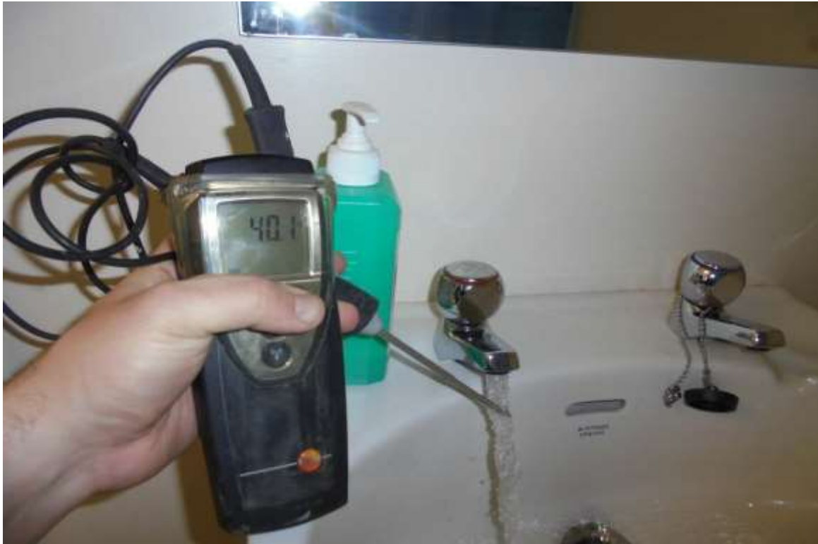
Public Toilet WHB – Hot Water Outlet Temperature Satisfactory – Thermostatic Control
