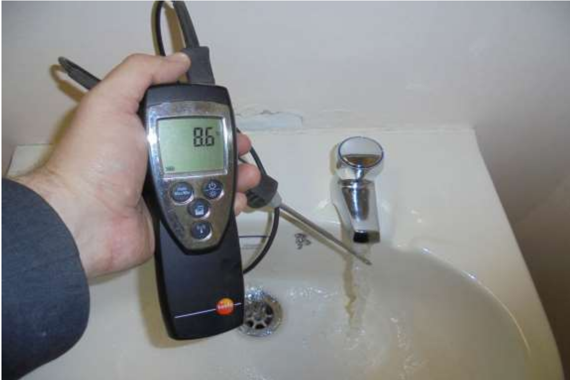
Public Toilet WHB - Cold Water Outlet Temperature Satisfactory
