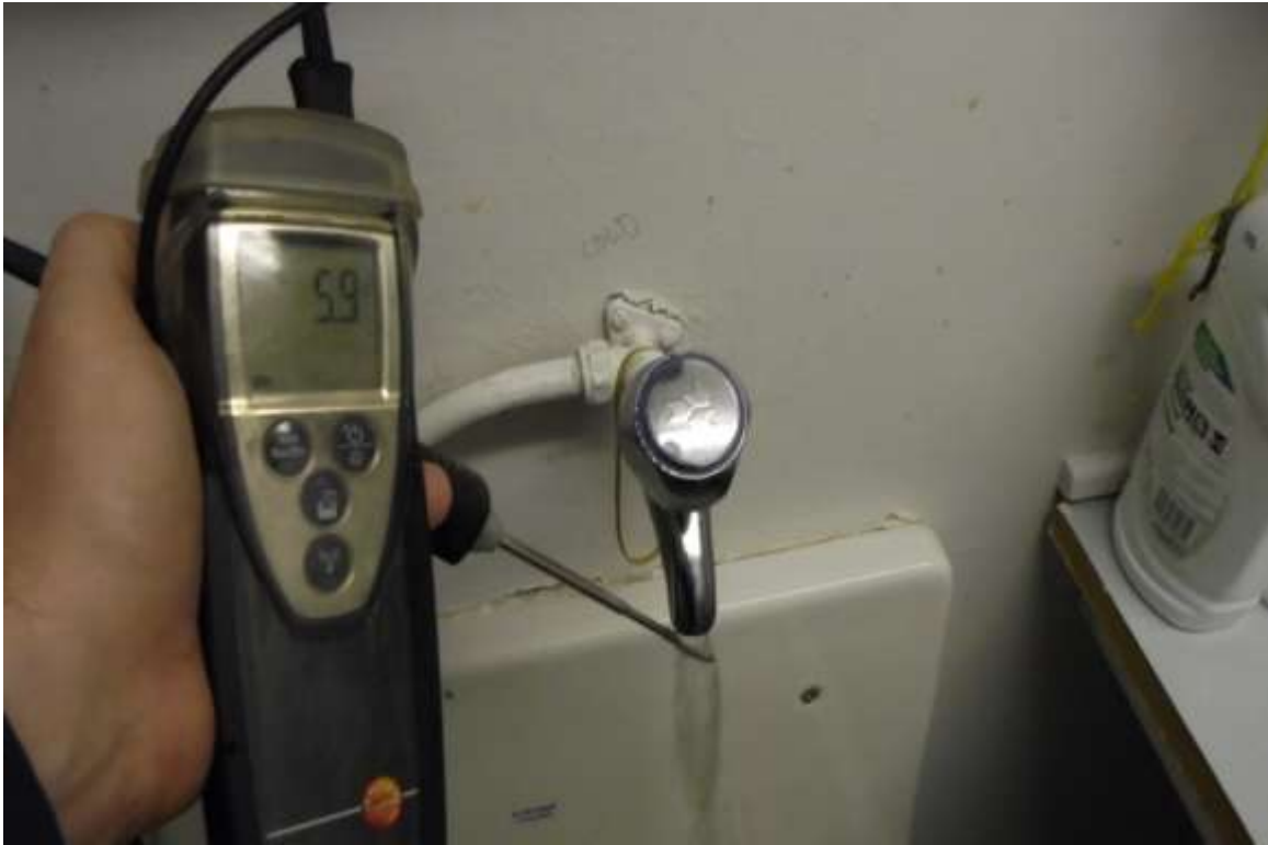
DRS Sink – Cold Water Outlet Temperature Satisfactory
