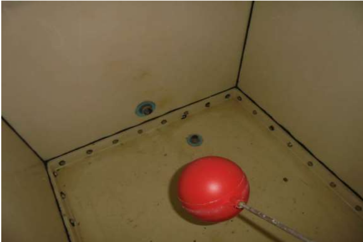
CWS Tank No. 2 – Drained and Isolated
