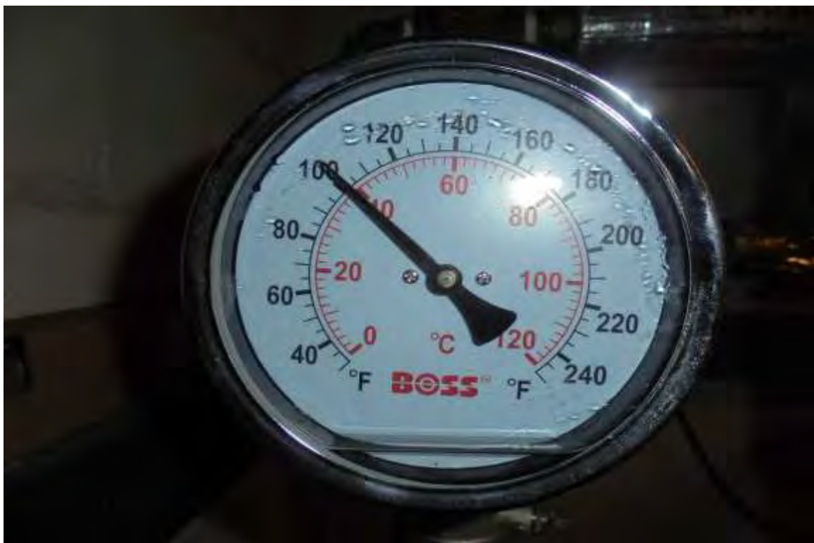
Gas Fired Water Heater No. 1 – Contents Temperature at Approximately 40°C Water in Gauge – Replace
