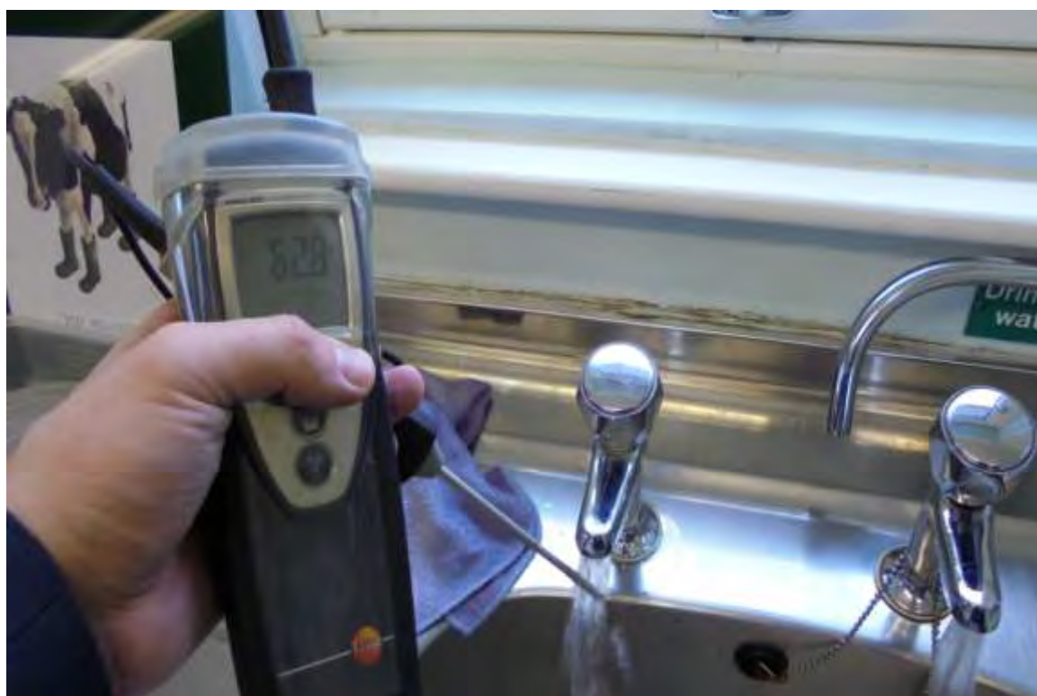
1 st Floor Staff Room Sink – Hot Water Outlet Temperature Too High (>60°C) Scald Hazard
