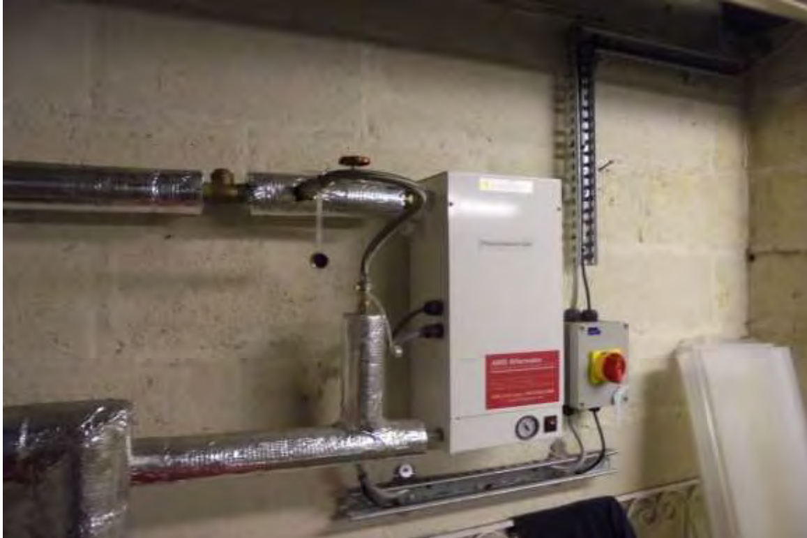
MWS Branch to Heating System Pressurisation Unit with Check Valve installed and Flexible Quick-fill Hose Connected
