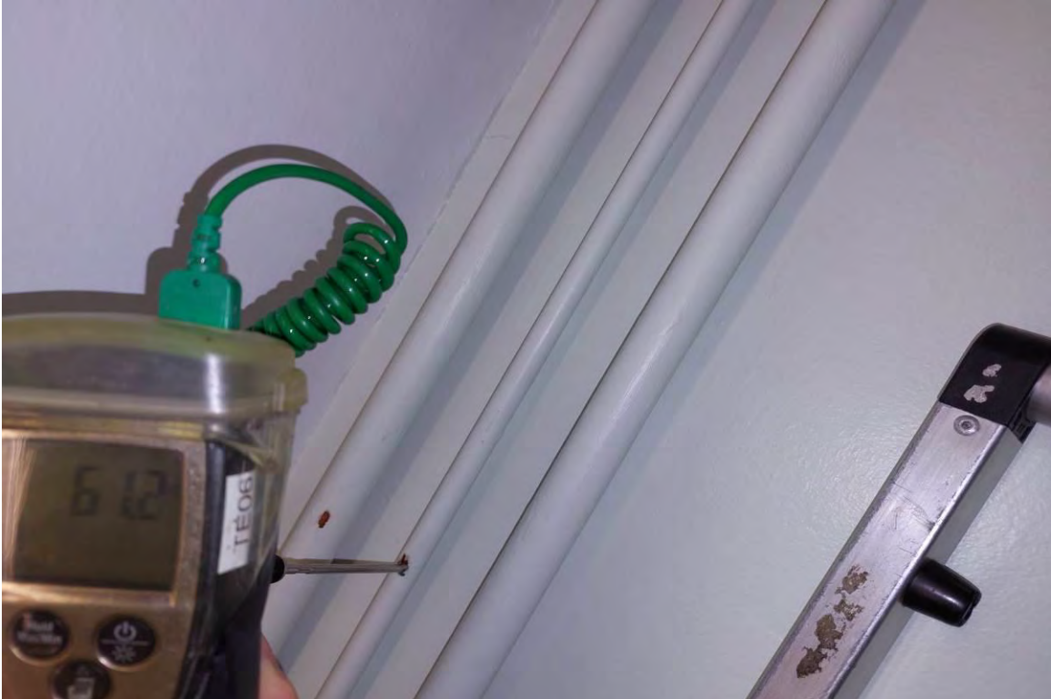
Return Temperature from Consultant Room 8 Satisfactory
