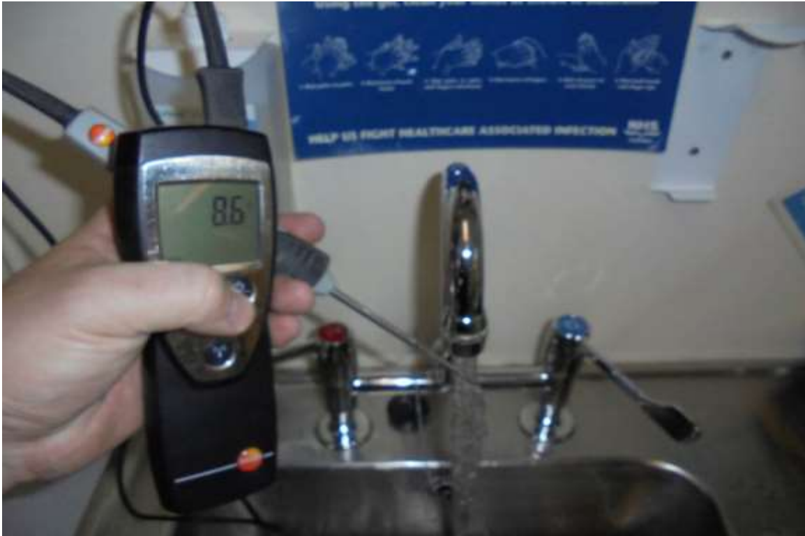
Health Education/Physio Room Sink – Cold Water Outlet Temperature Satisfactory
