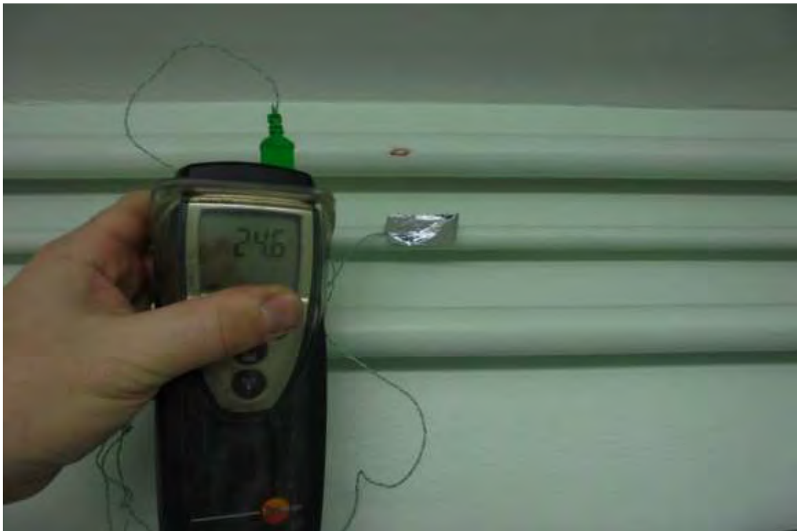
DHWS Return Temperature from Treatment Room G/49 Too Low (<55°C)
