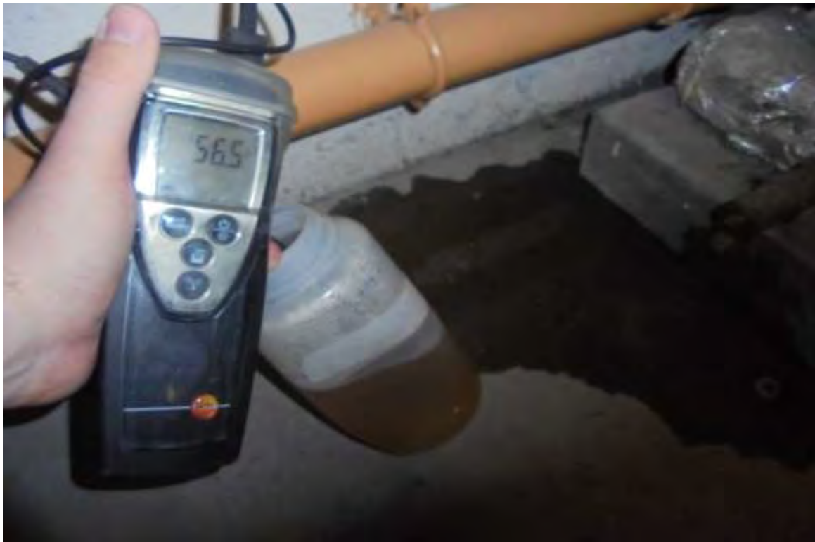
Gas Fired Water Heater No. 1 – Drain Sample Discoloured and at Satisfactory Temperature
