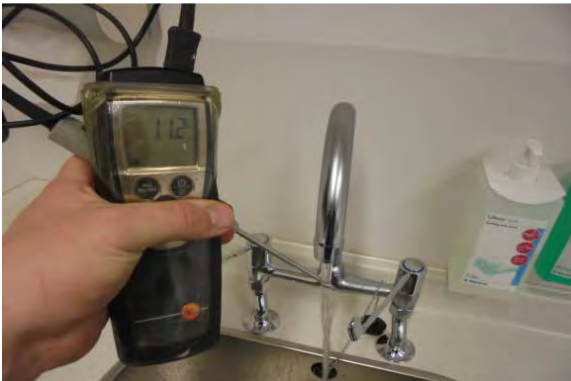
Extension Consulting Room 3 Sink – Hot Water Outlet Temperature Too Low (<50°C) Supplied via POUH
