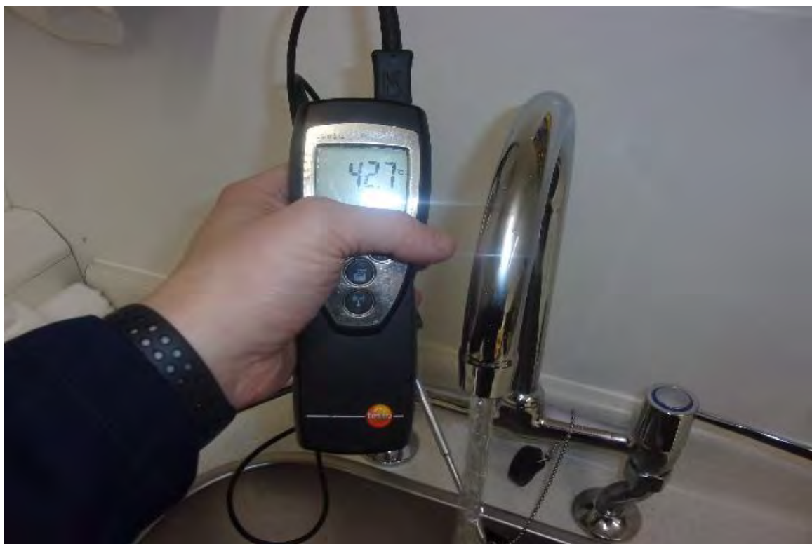
Consultant Room 1 (G/55) Sink – Hot Water Outlet Temperature Unsatisfactory (<50°C)
