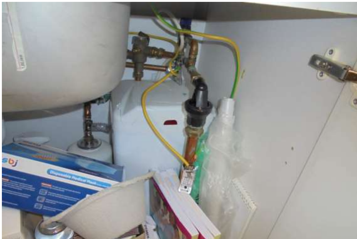
Extension Consultant Room 2 Under-Sink Electric Water Heater Provided
