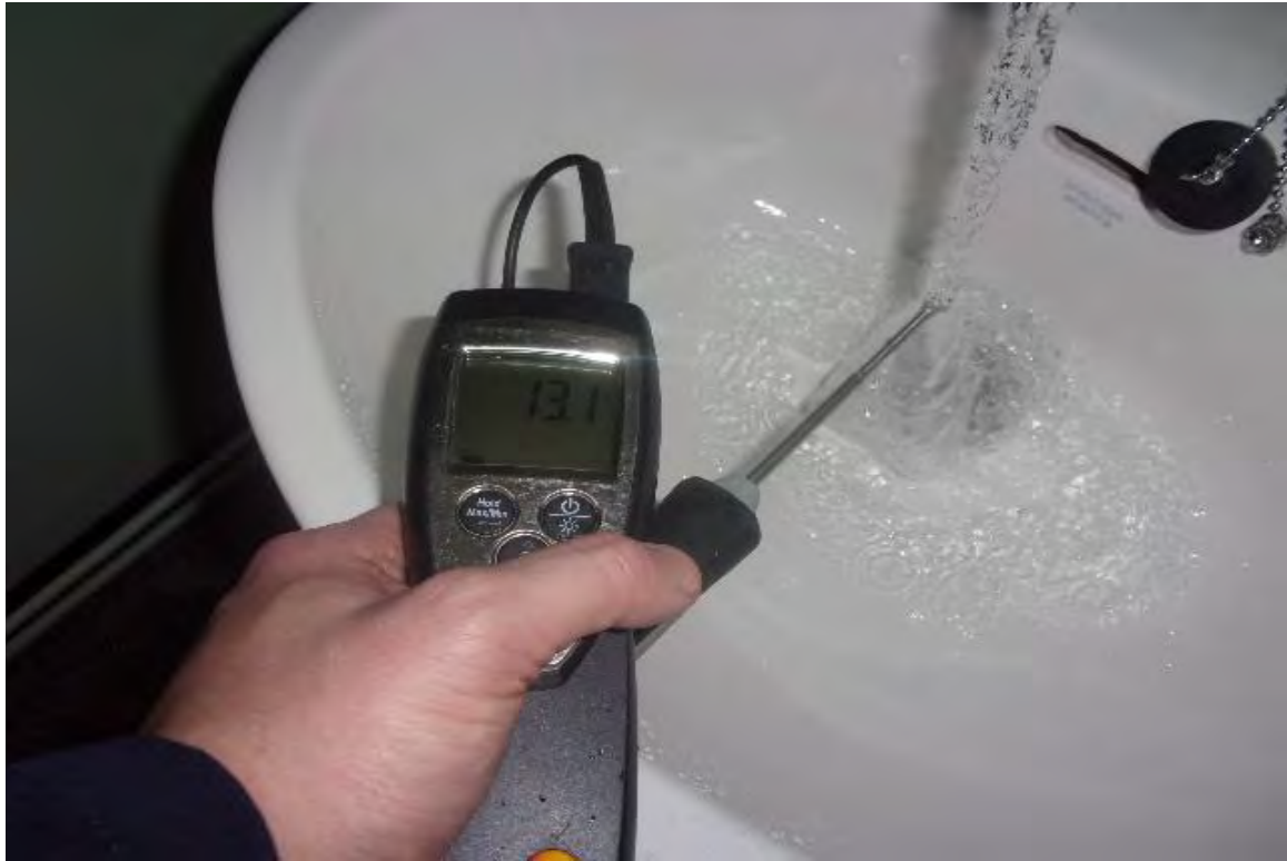
Consultant Room 2 (G/14) Sink - Cold Water Outlet Temperature Satisfactory
