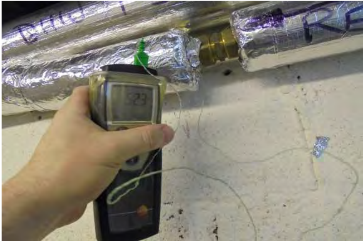
DHWS Return Temperature Too Low (<55°C)
