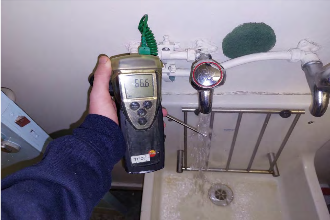
DSR Sink - Hot Water Outlet Temperature Satisfactory
