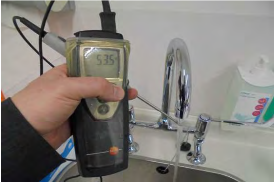
Extension Consulting Room 3 Sink - Hot Water Outlet Slightly Low (<50°C)
