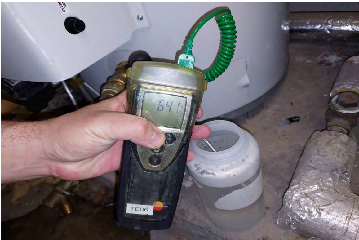
DHWS Gas Fired Water Heater No.1 – Drain Sample Light Sediment and at Satisfactory Temperature
