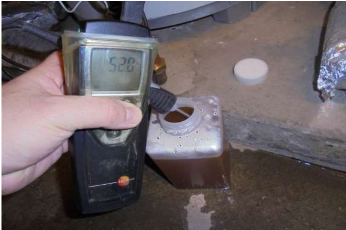
Gas Fired Water Heater No. 1 – Drain Sample Discoloured and at Acceptable Temperature
