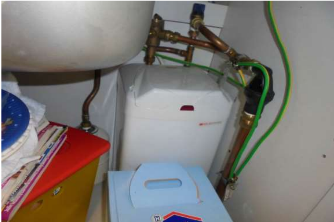
Extension Consulting Room 3 Sink – Electric Point of Use Water Heater
