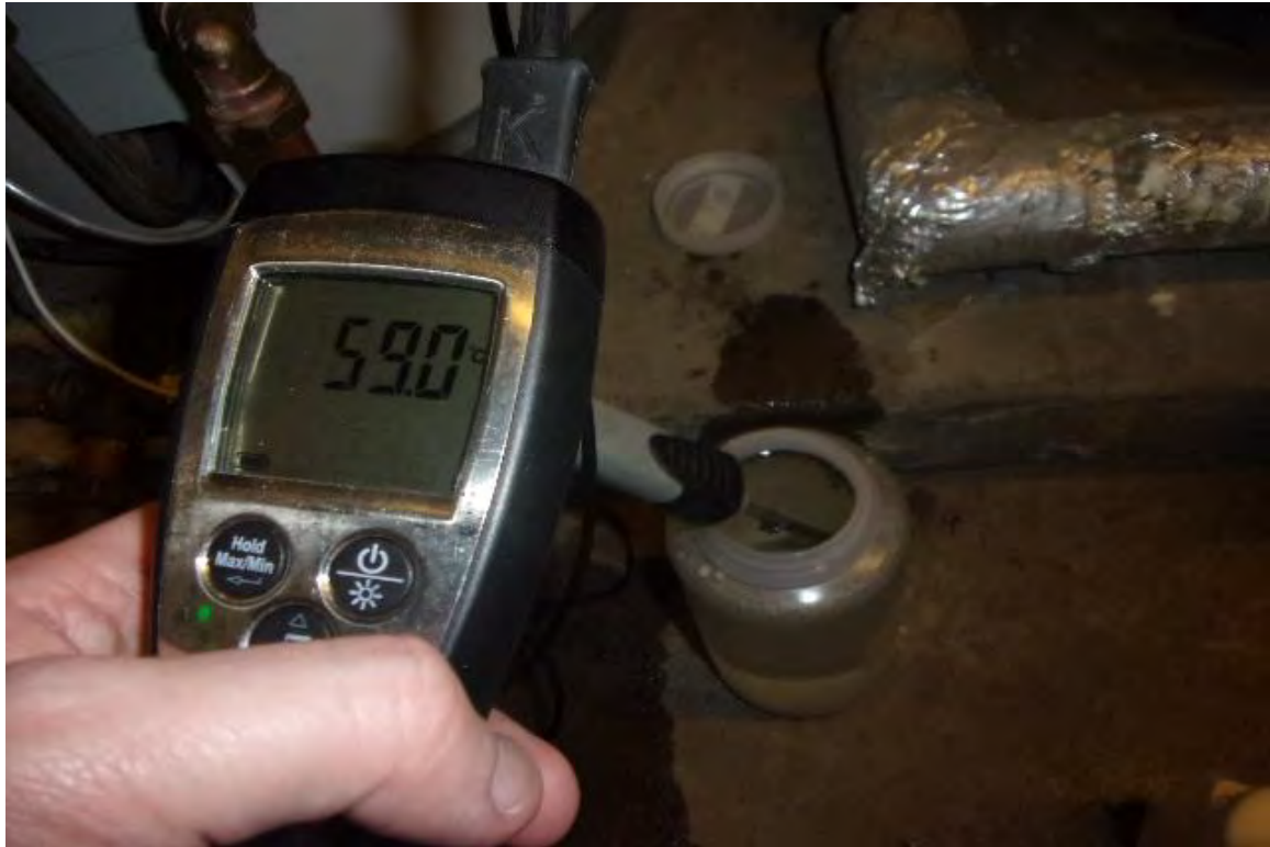
Gas Fired Water Heater No. 1 – Drain Sample Containing Light Sediment and at Satisfactory Temperature
