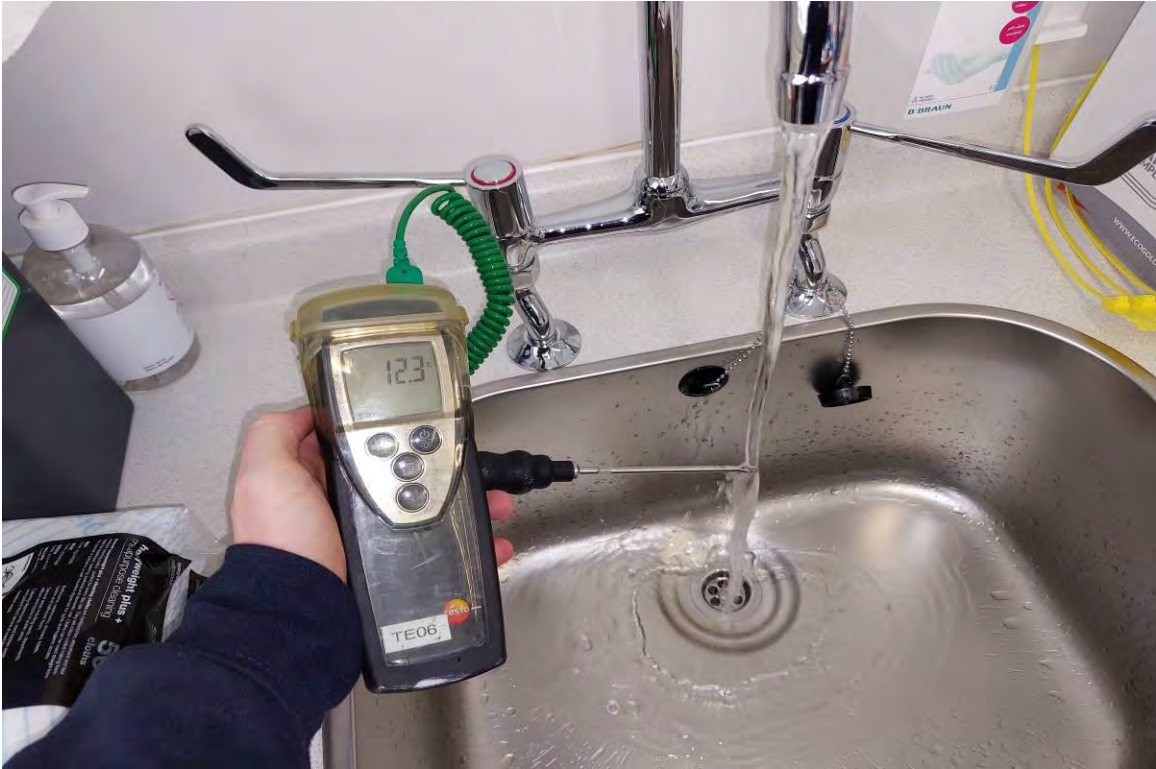
Extension Consultant Room 3 Sink - Cold Water Outlet Temperature Satisfactory
