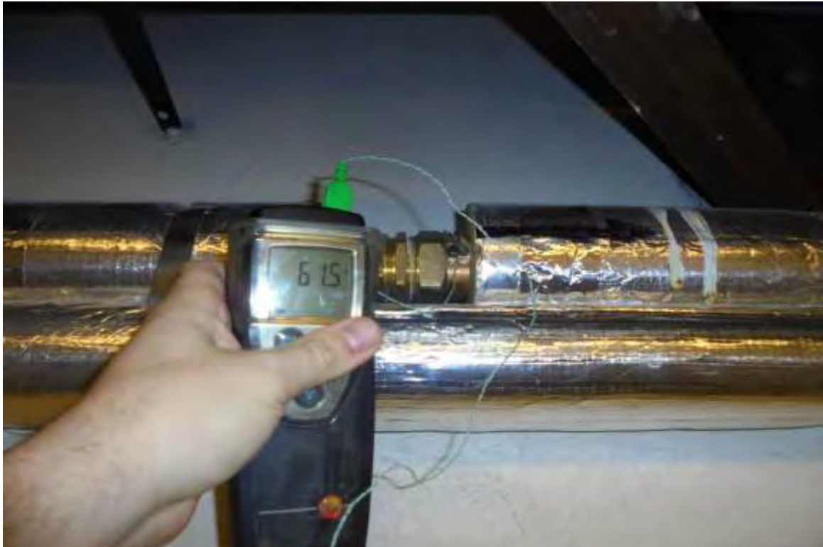
DHWS Flow Temperature Satisfactory (>55°C)
