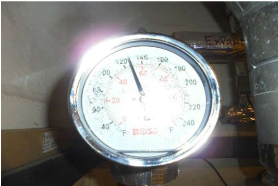
Gas Fired Water Heater No. 1 – Contents Gauge at 55°C
