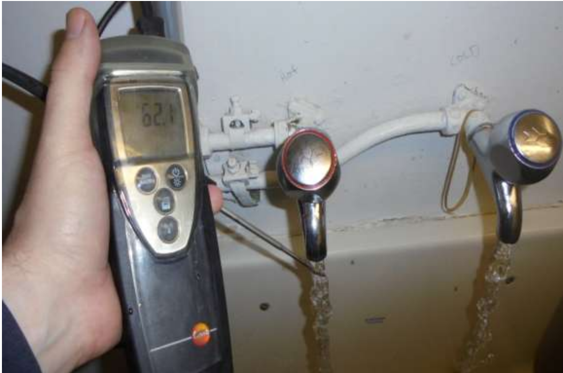
DRS Sink – Hot Water Outlet Temperature Too High (>60°C) Scald Hazard
