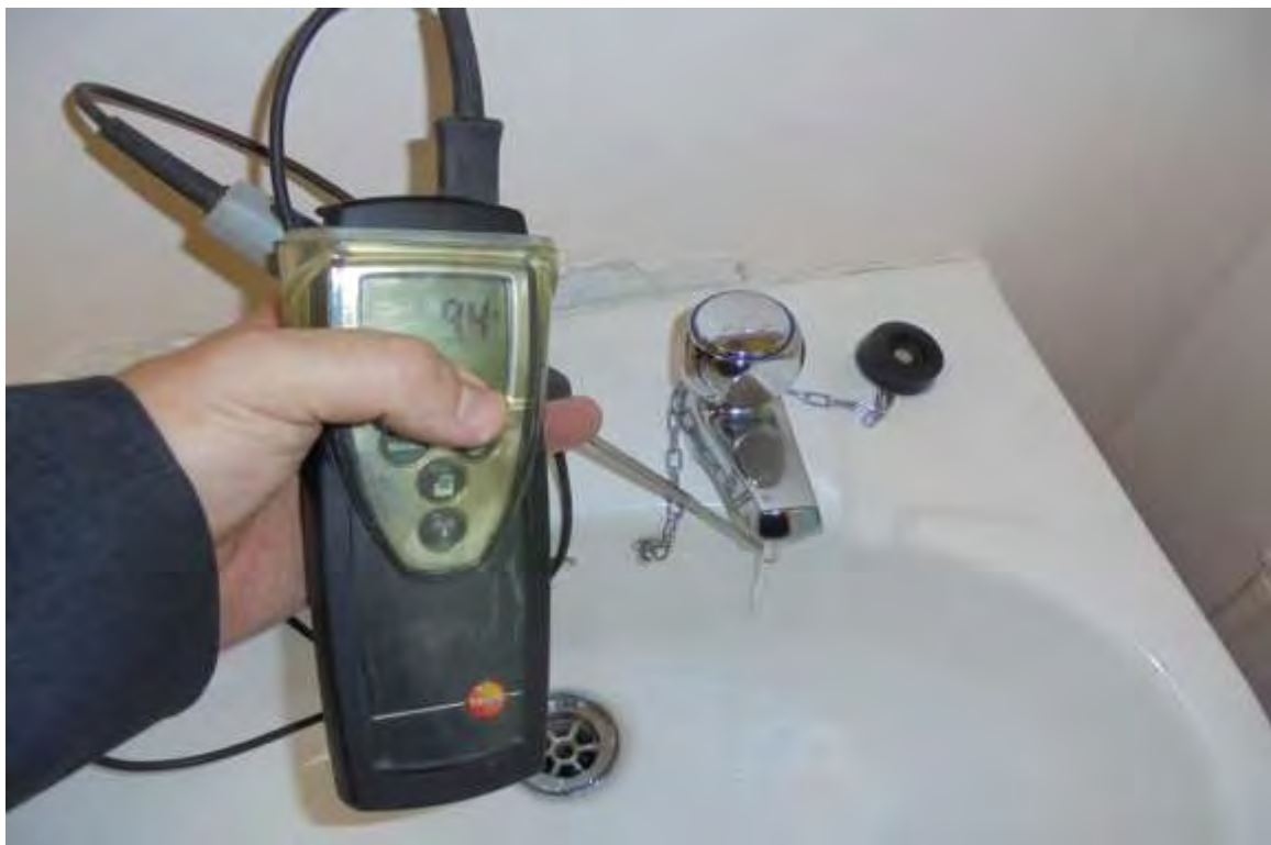
Reception Gents Toilet WHB - Cold Water Outlet Temperature Satisfactory
