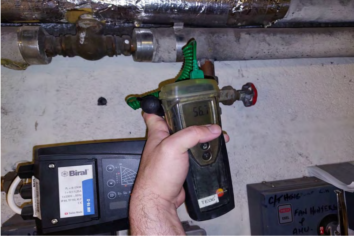
Plantroom Principle Loop Return Temperature Satisfactory
