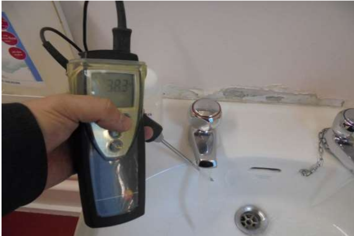
Patients Toilet G39 WHB – Hot Water Outlet Temperature Satisfactory Thermostatic Control
