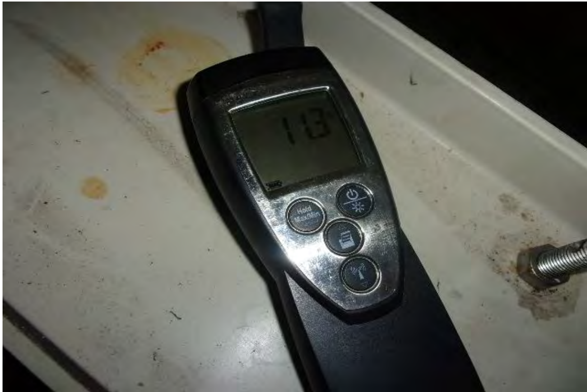
CWS Tank No. 1 – Contents Temperature at 11.5°C
