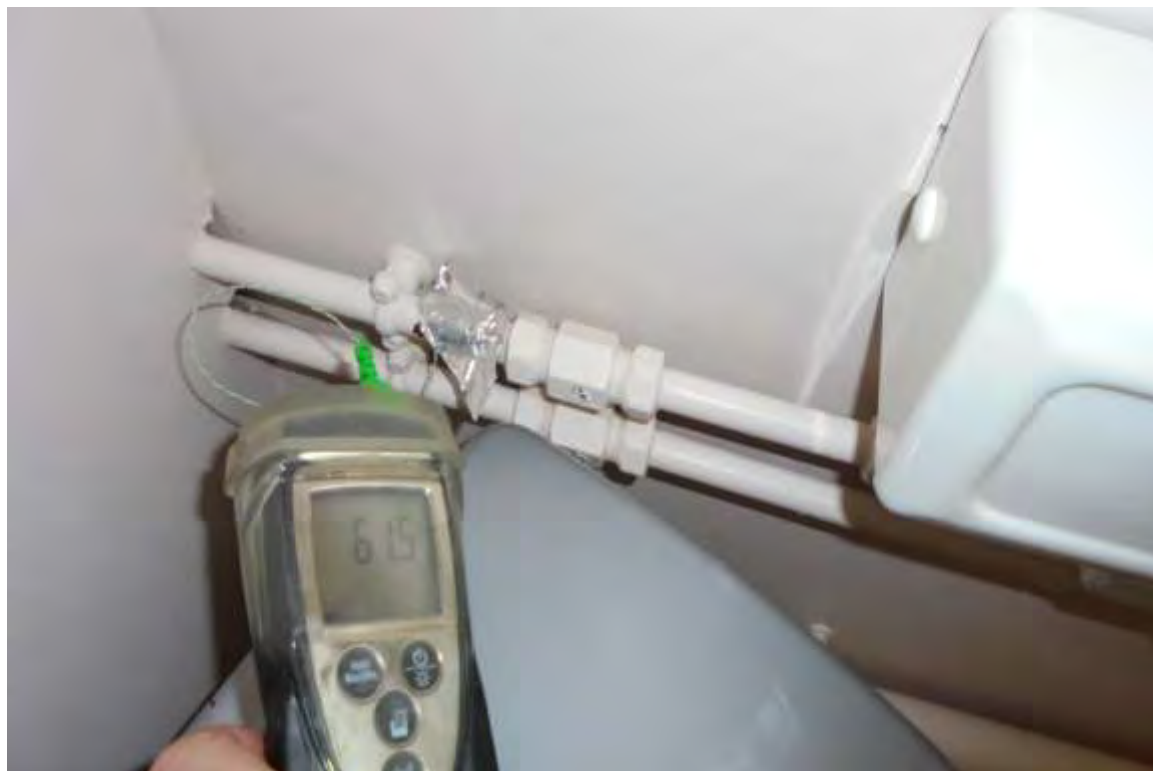
Public Toilet WHB – Hot Water Temperature to TMV Satisfactory
