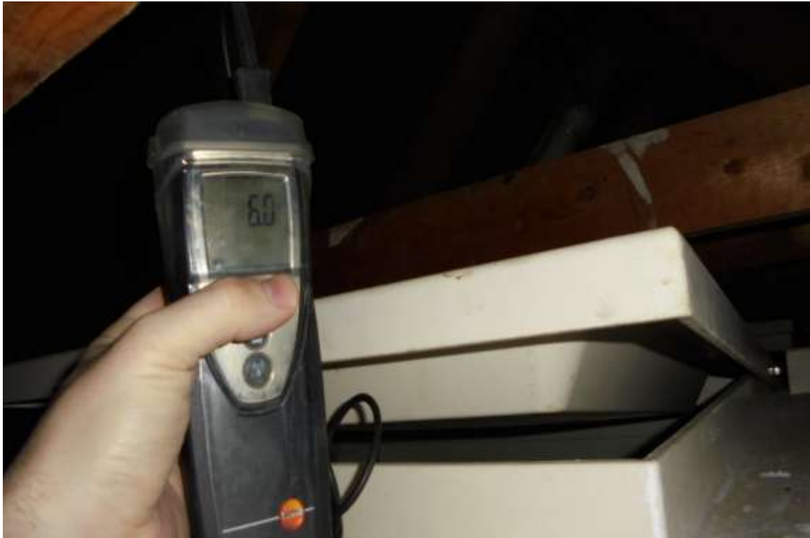
CWS Tank No. 1 – Contents Temperature Satisfactory
