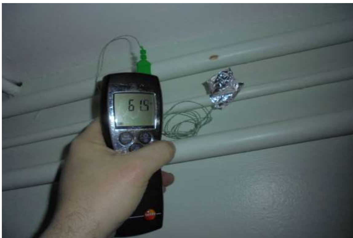
Return Temperature from Consultant Room 8 Satisfactory
