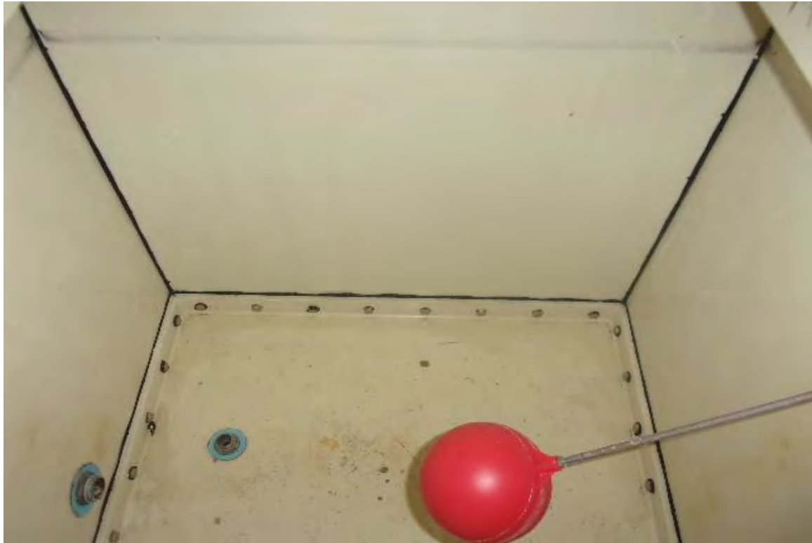
CWS Tank No. 2 – Drained and Isolated
