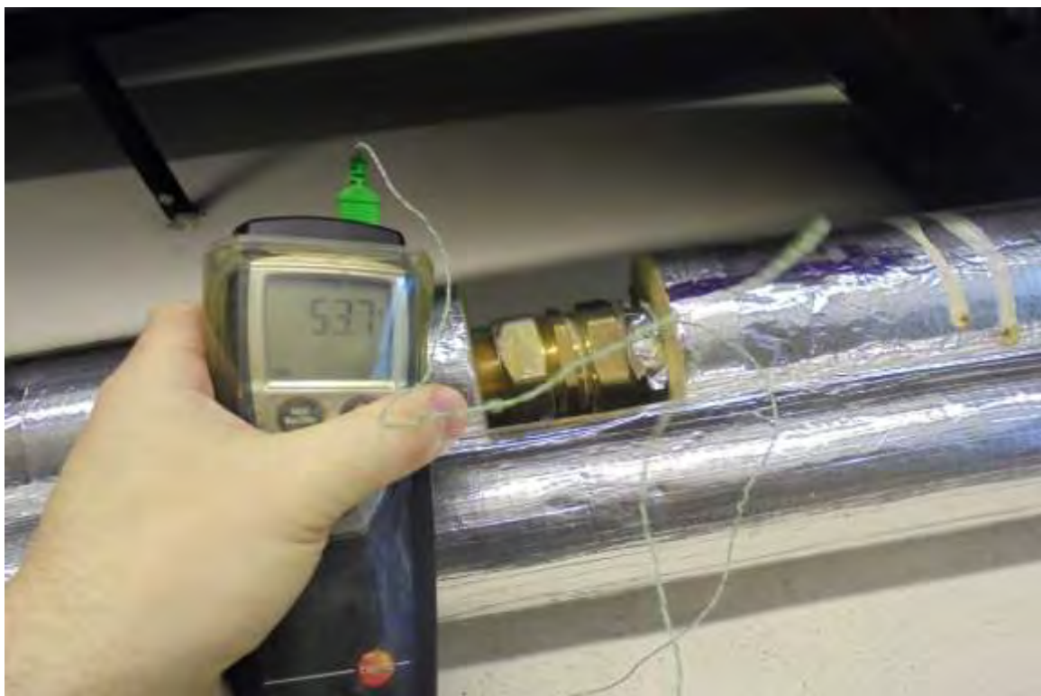
DHWS Flow Temperature Too Low (<60°C)
