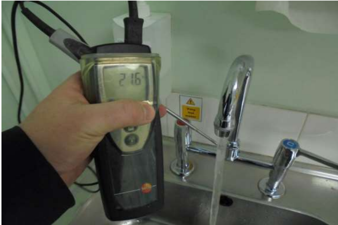
Room 8 (G/05) Sink - Hot Water Outlet Temperature Too Cold (<50°C)
