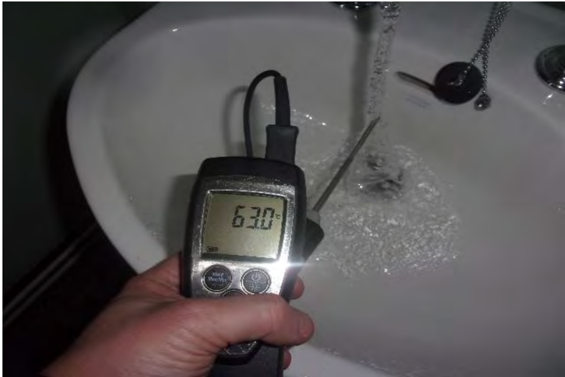
Consultant Room 2 (G/14) Sink - Hot Water Outlet Temperature Satisfactory
