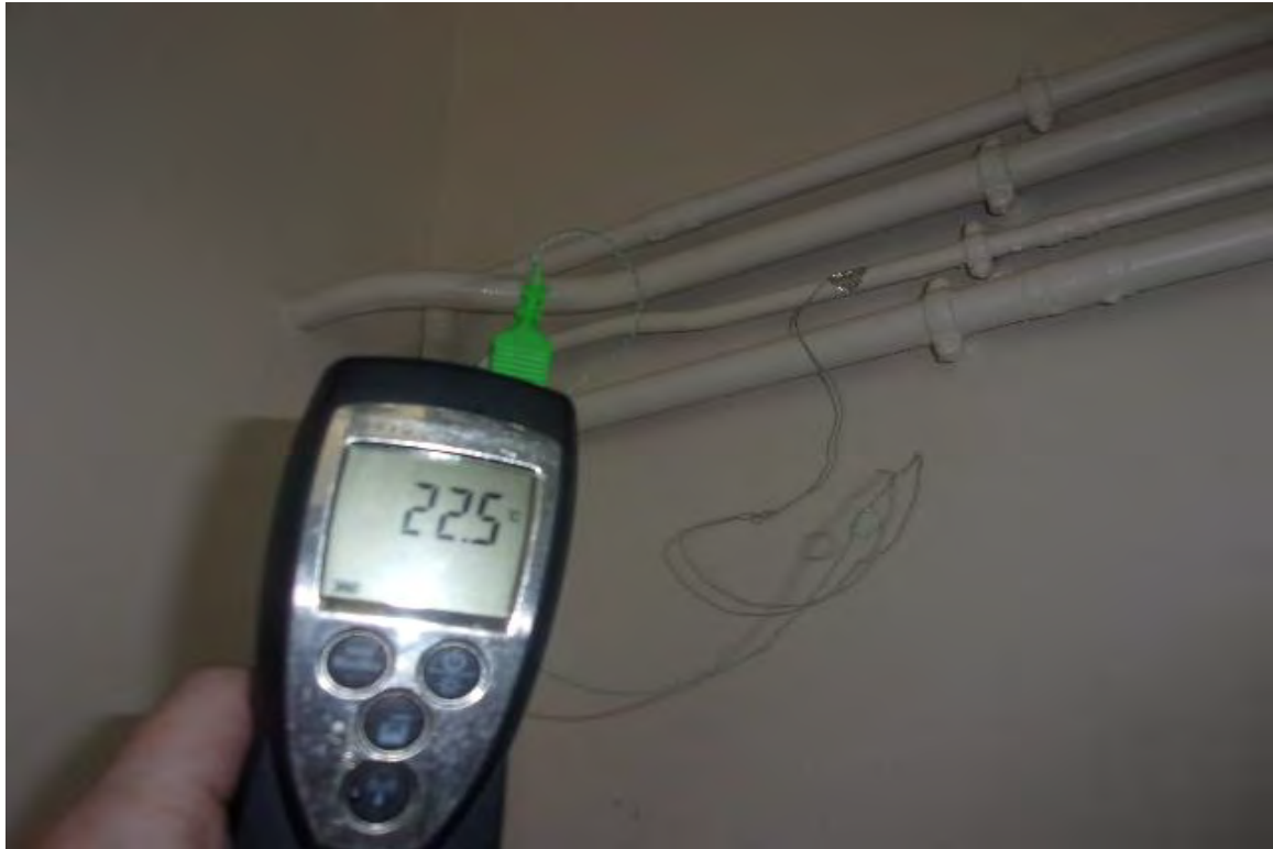
Baby Changing Area Hot Water Return Temperature Too Low (<55°C)
