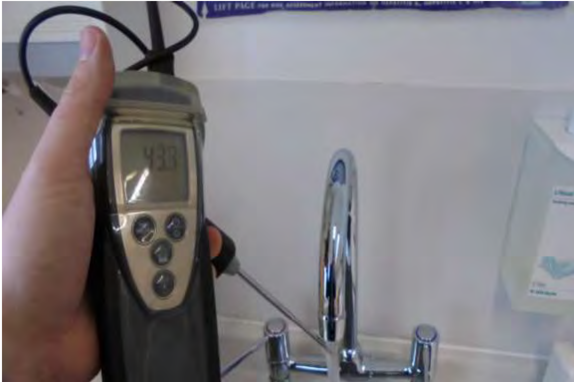
Extension Consulting Room 3 Sink – Hot Water Outlet Temperature Too Low (<50°C) Supplied via POUH
