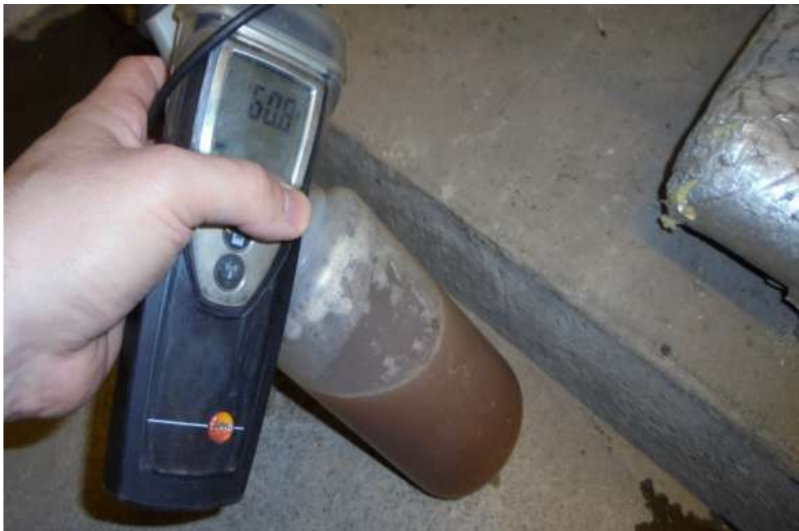
Gas Fired Water Heater No. 2 – Drain Sample Discoloured and at Satisfactory Temperature
