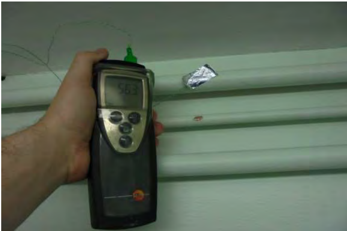
DHWS Flow Temperature to Treatment Room G/49 Satisfactory after Extended Flush
