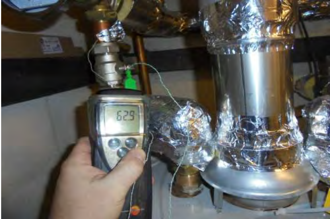
Gas Fired Water Heater No. 1 – Contents Temperature Confirmed at 63°C
