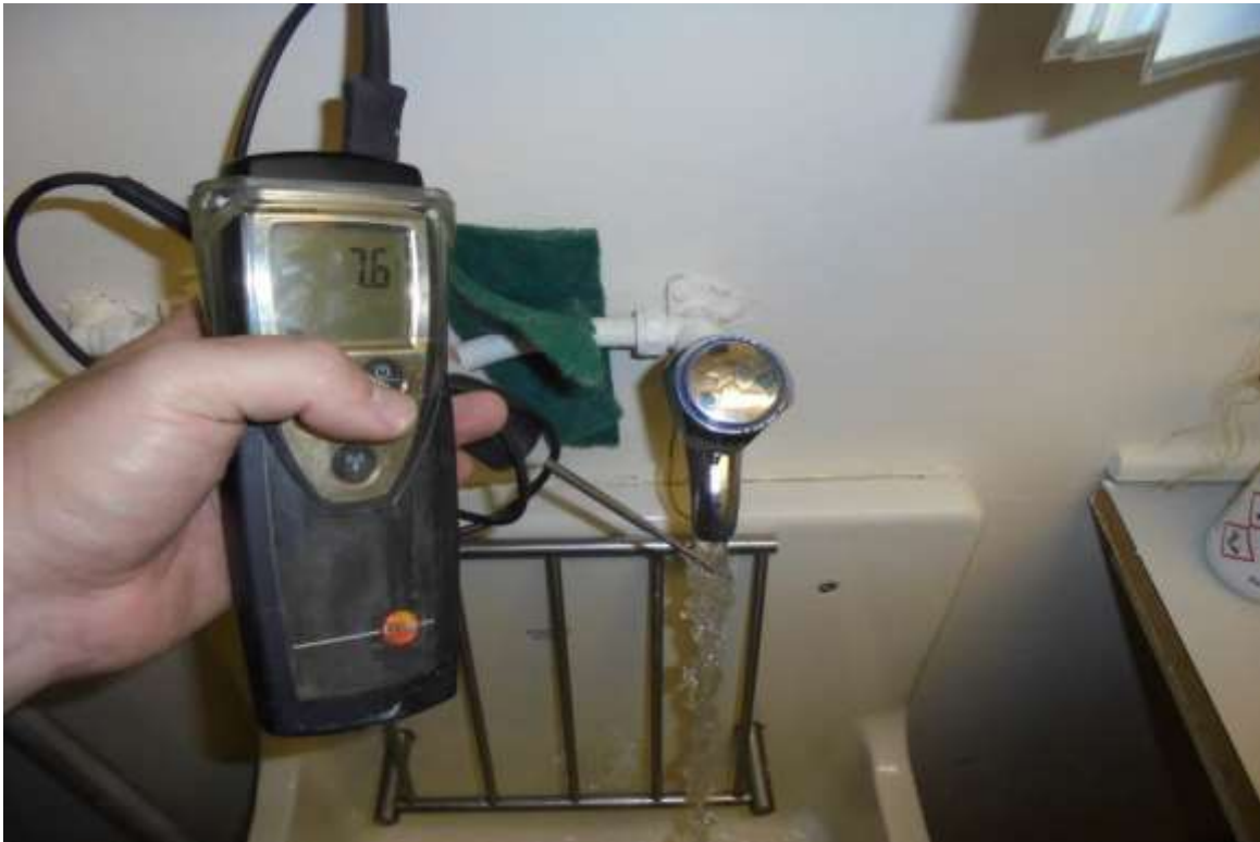
DRS Sink – Cold Water Outlet Temperature Satisfactory
