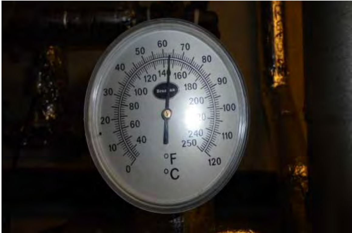
Gas Fired Water Heater No. 2 – Contents Gauge at 62°C
