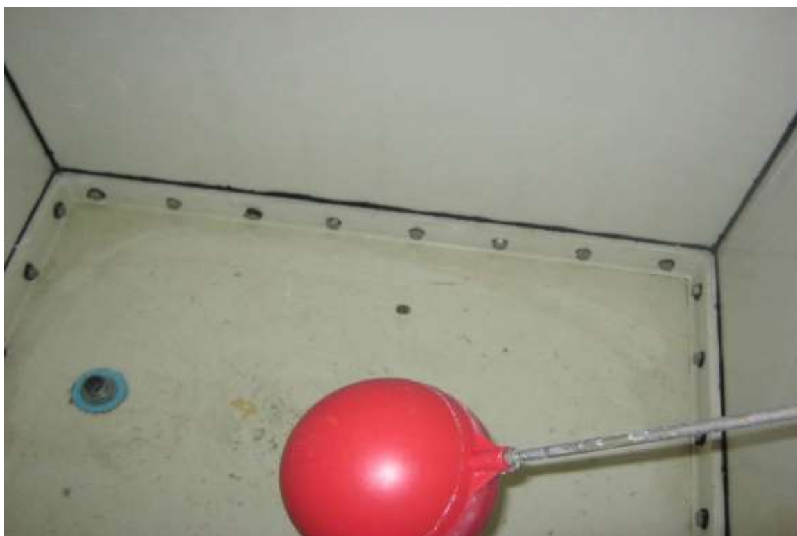
CWS Tank No. 2 – Drained and Isolated
