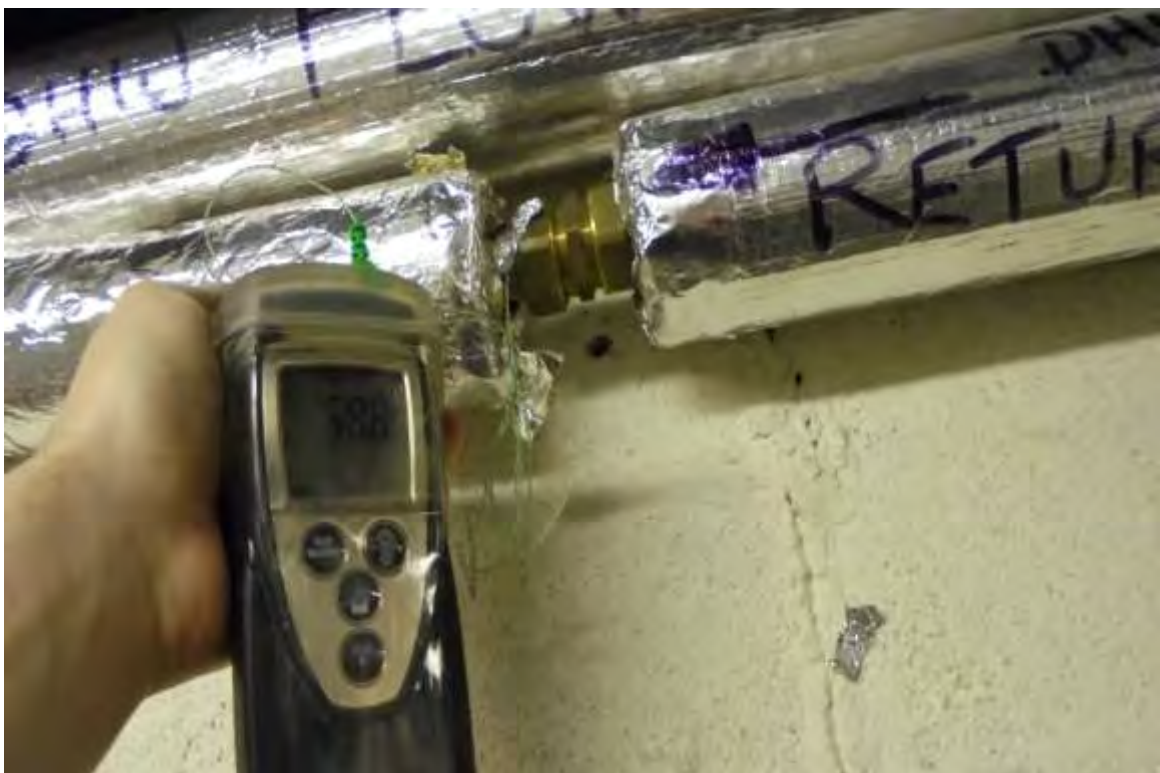
DHWS Return Temperature Satisfactory (>55°C)
