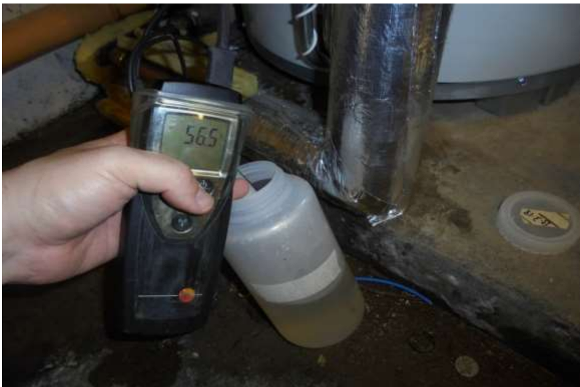
Gas Fired Water Heater No. 1 – Drain Sample Clear and at Satisfactory Temperature
