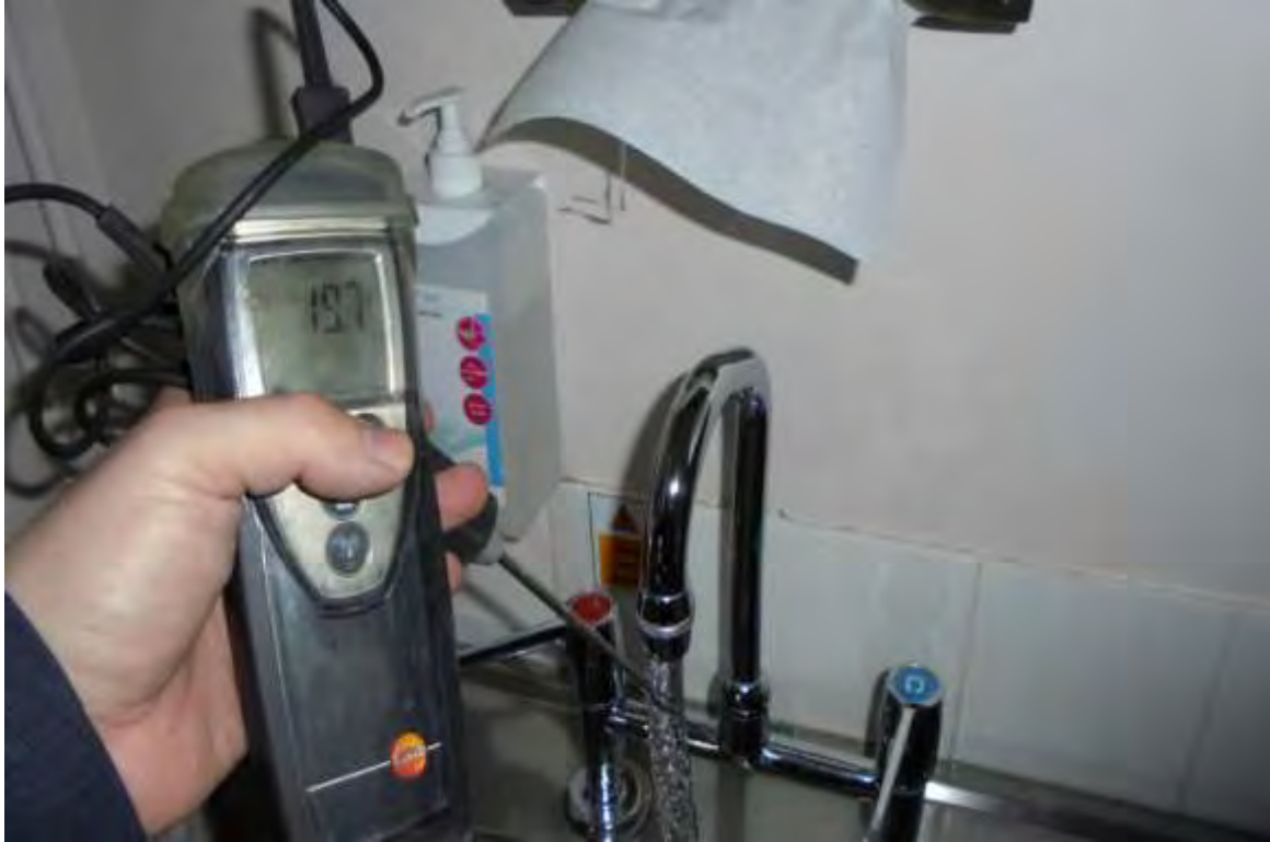
Treatment Room G/49 Sink – Hot Water Too Low After 1 Minute (<55°C)
