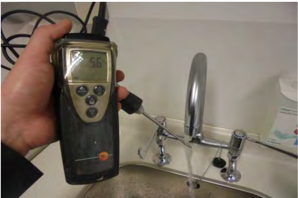
Extension Consulting Room 3 Sink – Cold Water Outlet Temperature Satisfactory
