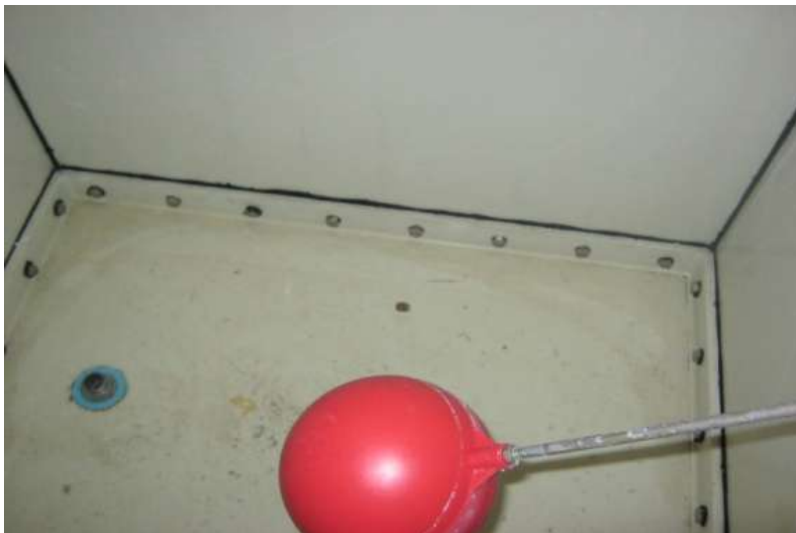
CWS Tank No. 2 – Drained and Isolated
