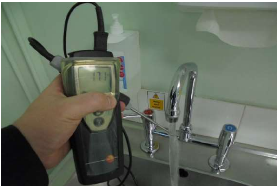
Room 8 (G/05) Sink - Cold Water Outlet Temperature Too Warm ( >20^{\circ}\text{C} )
