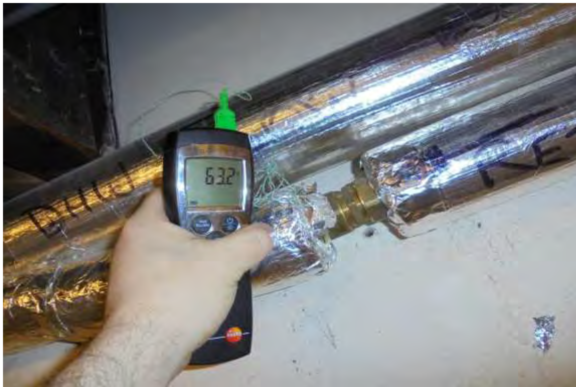
Plantroom Principle Loop Return Temperature Satisfactory
