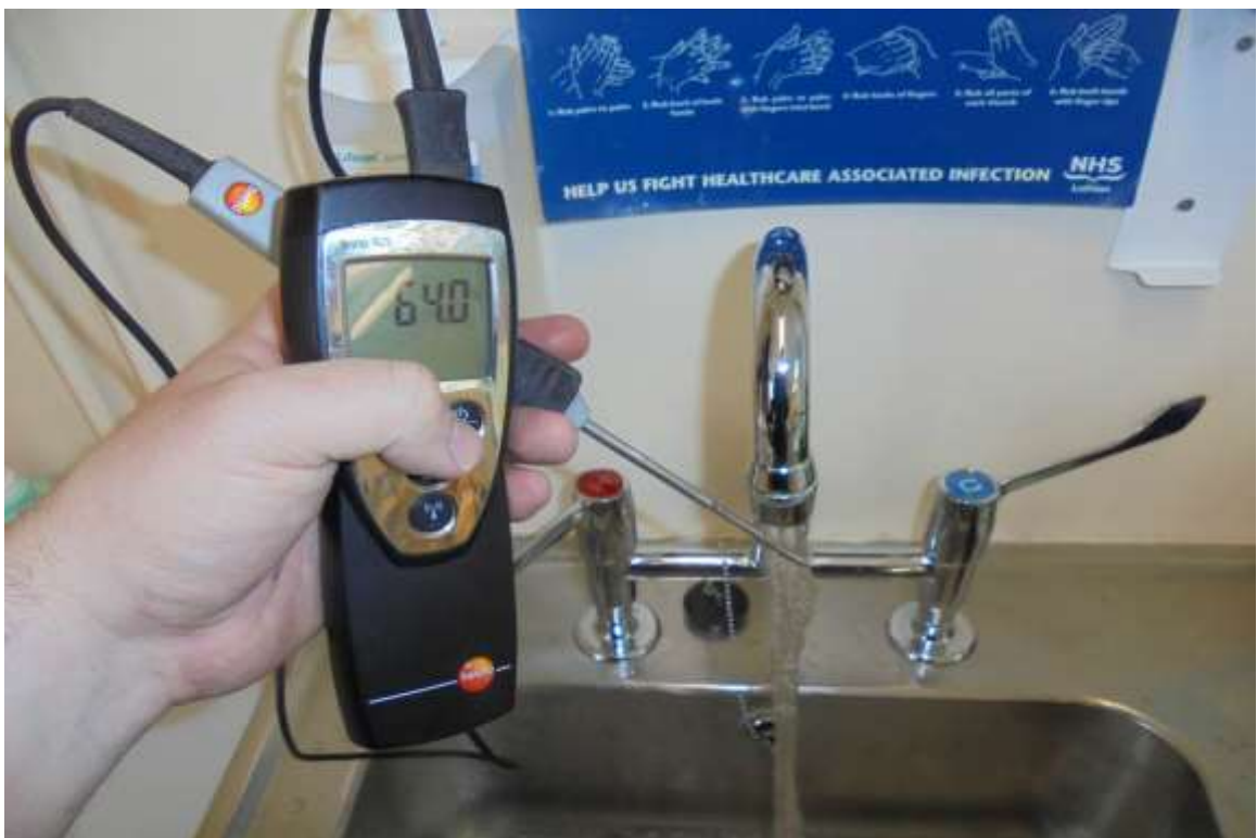
Health Education/Physio Room Sink - Hot Water Outlet Temperature Satisfactory
