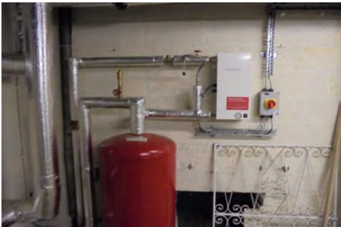
MWS Branch to Heating System Pressurisation Unit with Check Valve installed at Connection to Pressurisation Unit
