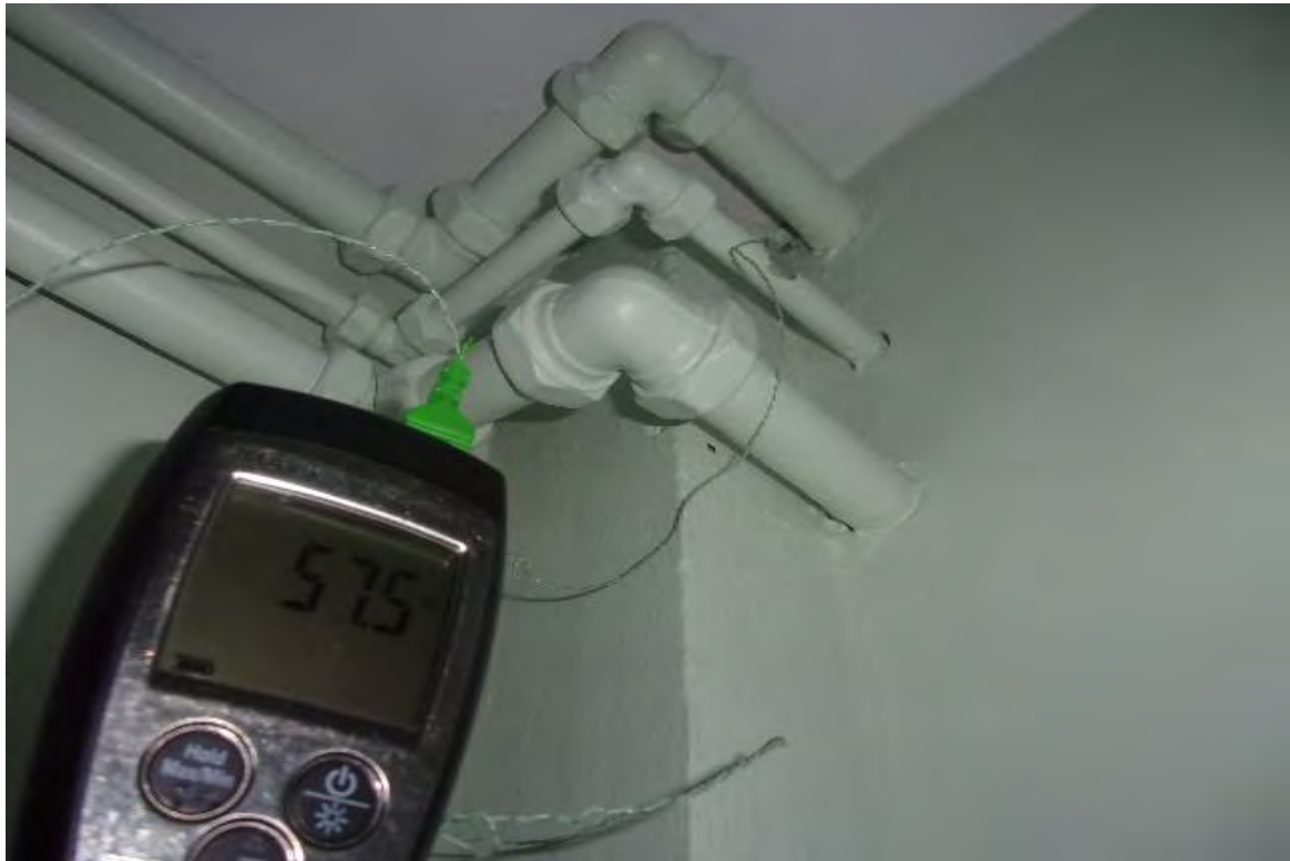
Secretarial Office (G/09) Hot Water Return Temperature Satisfactory
