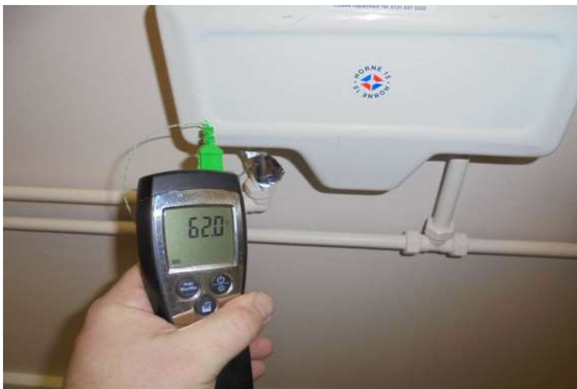
Public Toilet WHB - Supply Temperature to TMV Satisfactory (>55°C)
