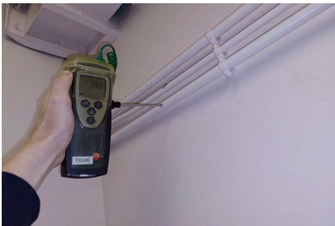
Health Education/Physio Room - Tertiary Loop Flow Temperature Too Low (<55°C)
