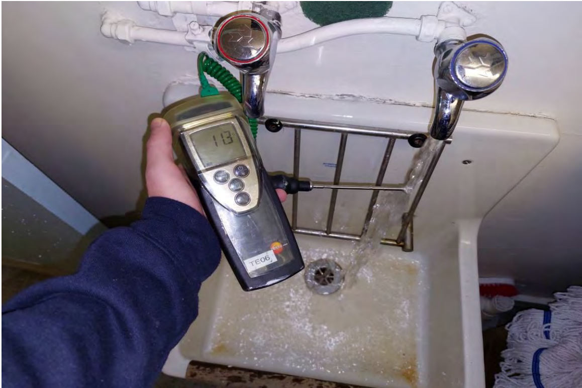
DSR Sink – Cold Water Outlet Temperature Satisfactory
