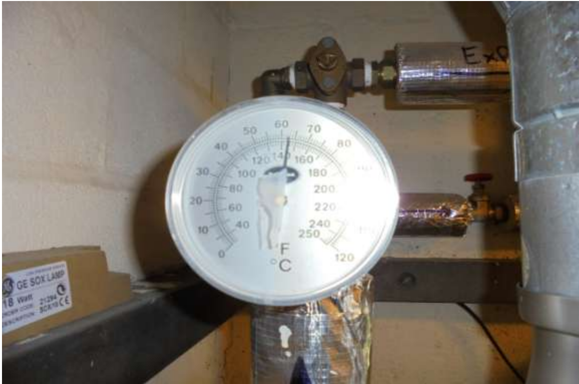
Gas Fired Water Heater No. 1 – Contents Gauge at 62°C
