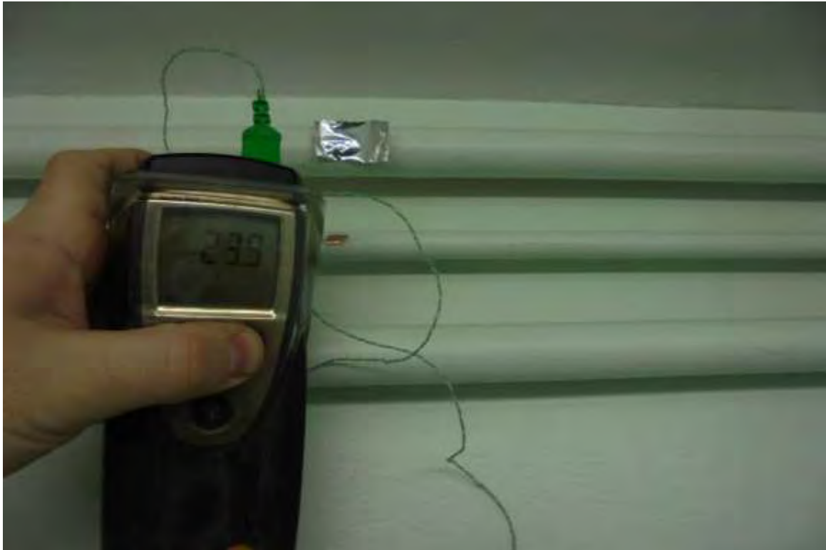
DHWS Flow Temperature to Treatment Room G/49 Too Low (<55°C)
