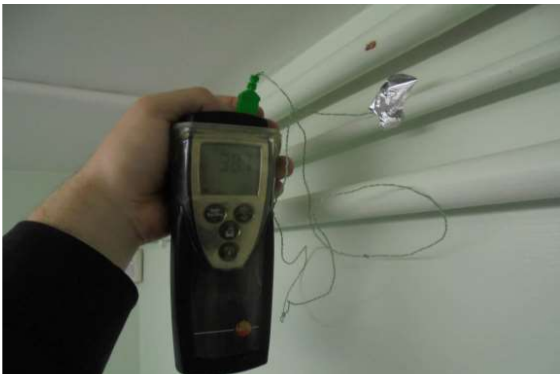
Secretarial Office (G/09) Hot Water Return Temperature Too Low (<55°C)
