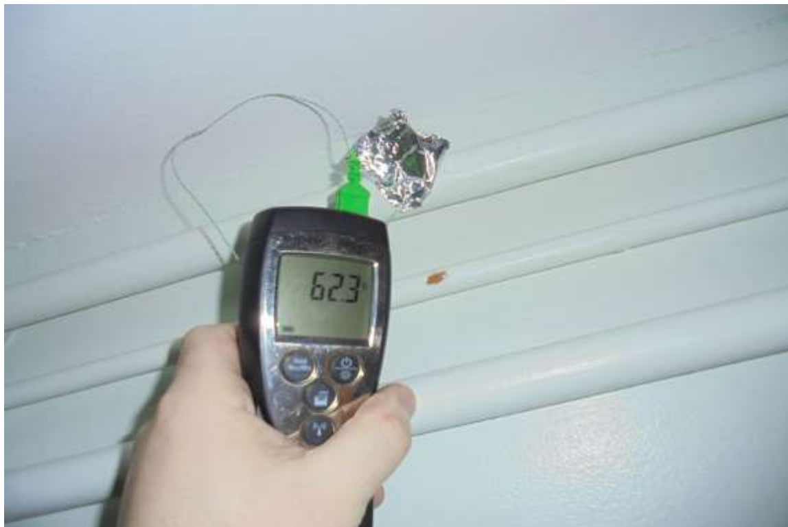
Flow Temperature to Consultant Room 8 Satisfactory
