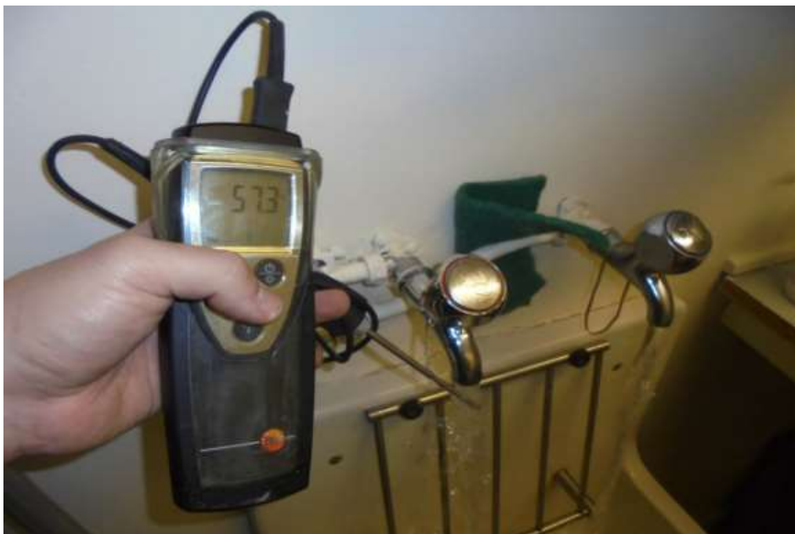
DRS Sink – Hot Water Outlet Temperature Satisfactory
