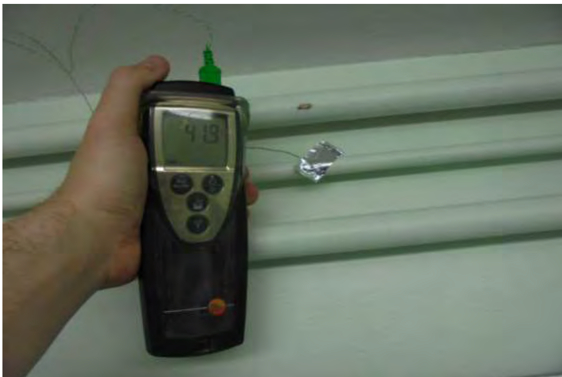
DHWS Return Temperature from Treatment Room G/49 Too Low (<55°C) after Extended Flush
