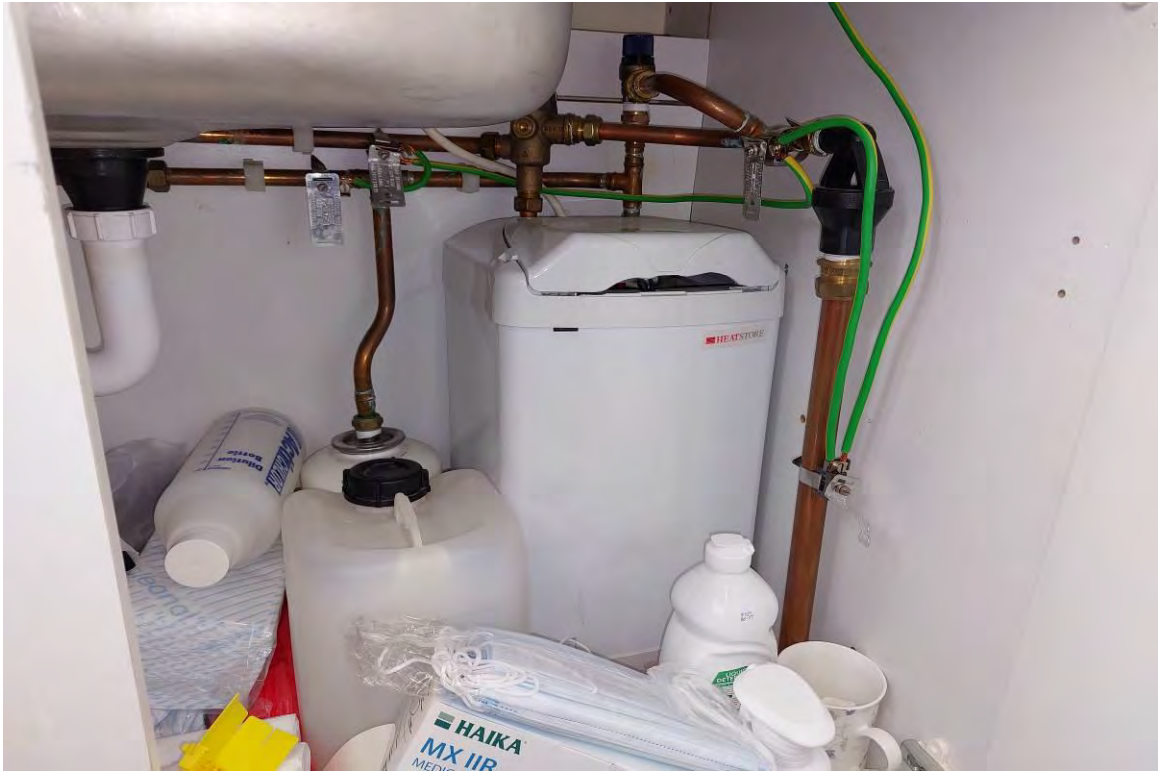
Extension Consultant Room 3 Under-Sink Electric Water Heater Provided
