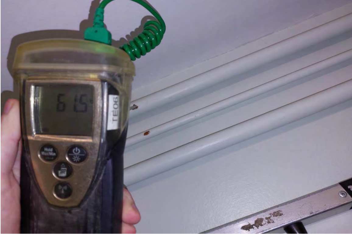
Flow Temperature to Consultant Room 8 Satisfactory
