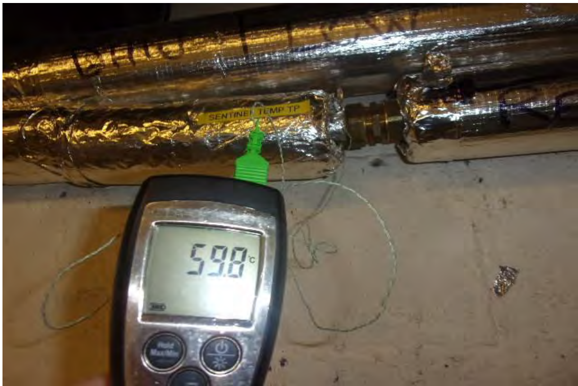
Plantroom Return Temperature Satisfactory
