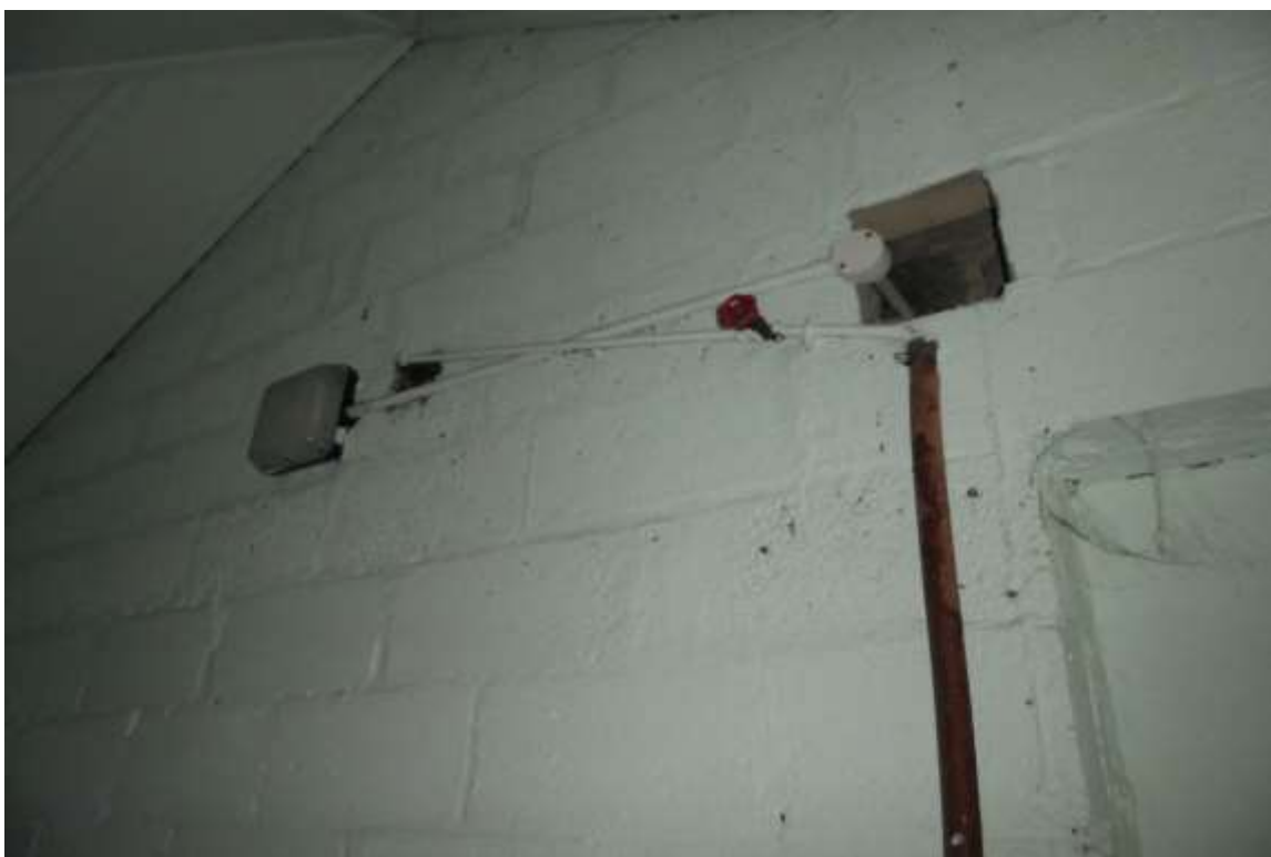
Bin Store MWS Connection Isolated at High Level – Effective Dead Leg
