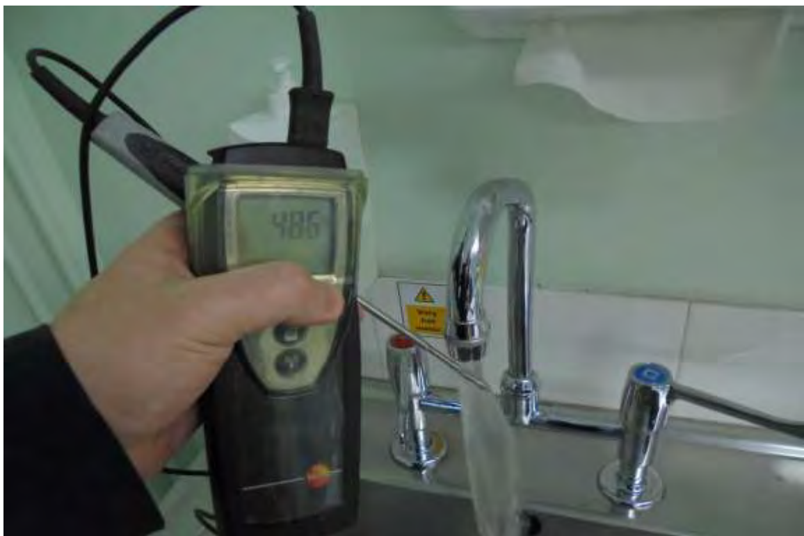
Room 8 (G/05) Sink - Hot Water Outlet Temperature Too Low (<50°C) After Extended Flush (4 Minutes)
