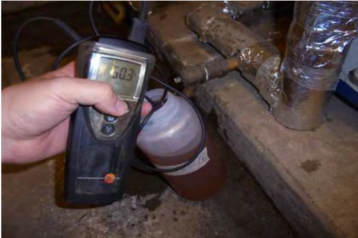
Gas Fired Water Heater No. 2 –Drain Sample Discoloured and at Satisfactory Temperature
