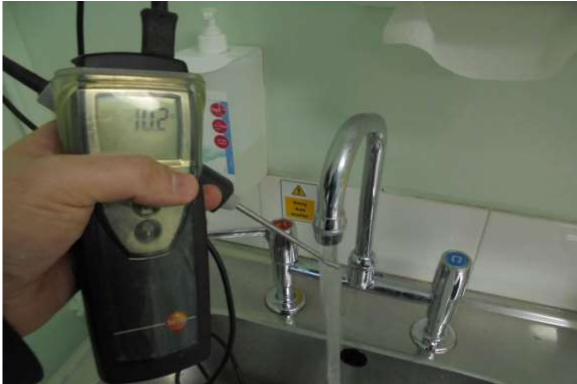
Room 8 (G/05) Sink - Cold Water Outlet Temperature Satisfactory After Extended Flush (4 Minutes)
