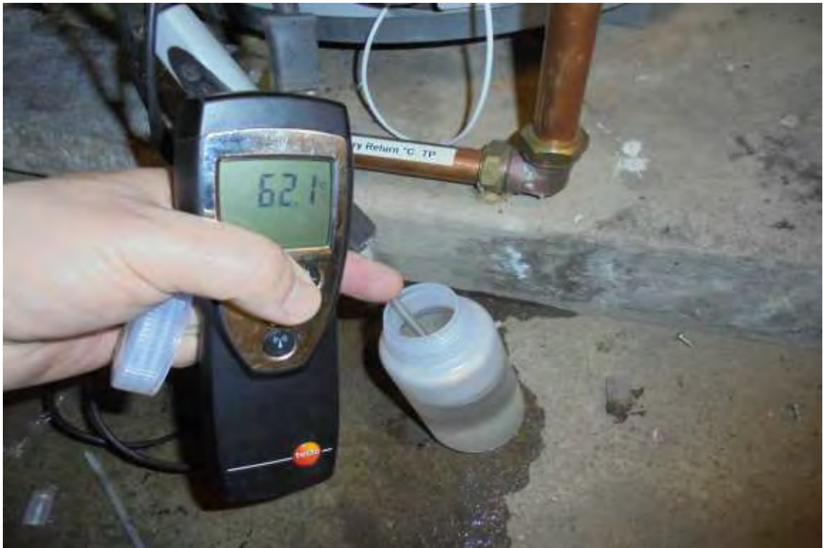
DHWS Gas Fired Water Heater No.1 – Drain Sample Clear and at Satisfactory Temperature
