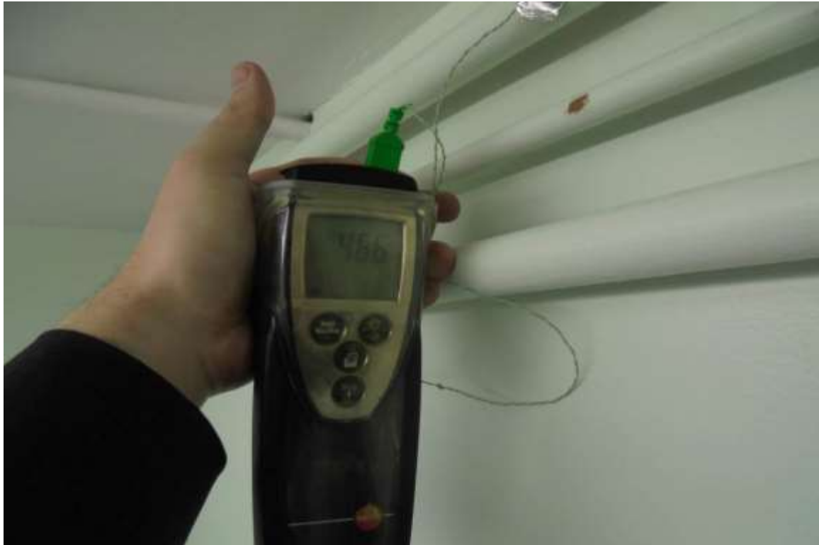
Secretarial Office (G/09) Hot Water Flow Temperature Too Low (<55°C)
