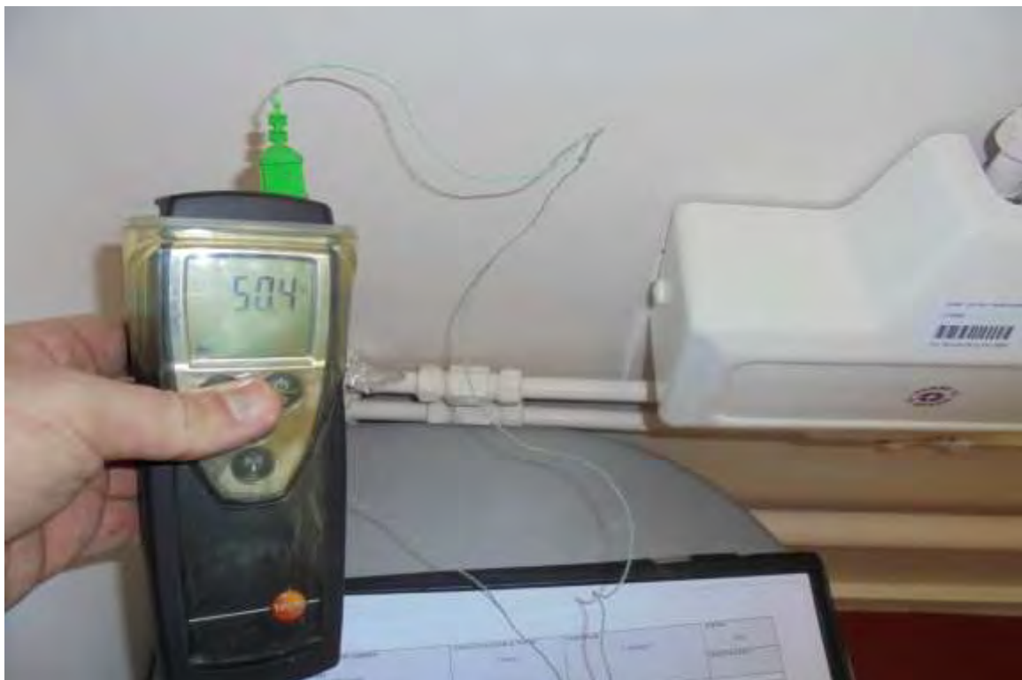
Reception Gents Toilet WHB – Supply Temperature to TMV Too Low (<55°C)
