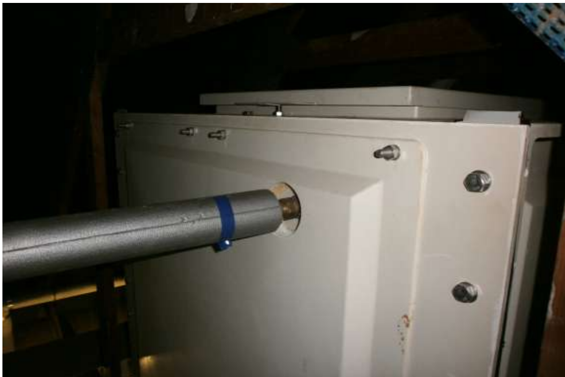
Roofspace CWS Tank – Pre Insulated GRP Construction
