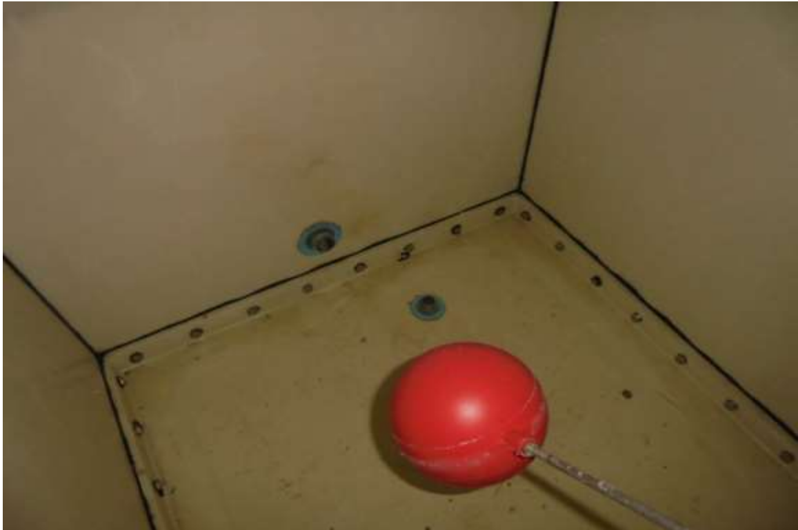
CWS Tank No.1 – Drained and Isolated
