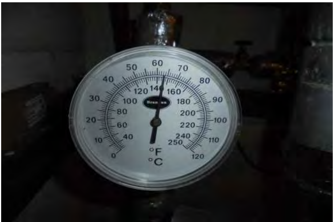
DHWS Gas Fired Water Heater No.1 - Storage Temperature Approximately 65°C
