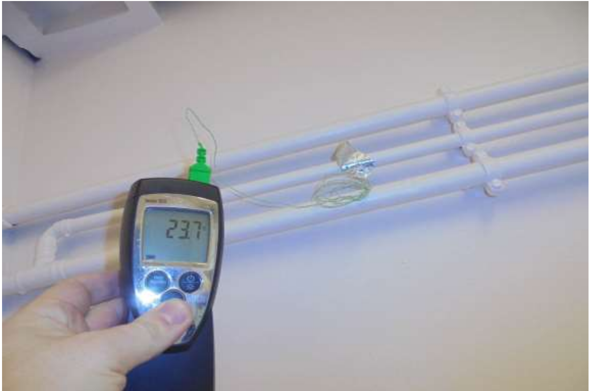
Health Education/Physio Room - Tertiary Loop Return Temperature Too Low (<55°C)
