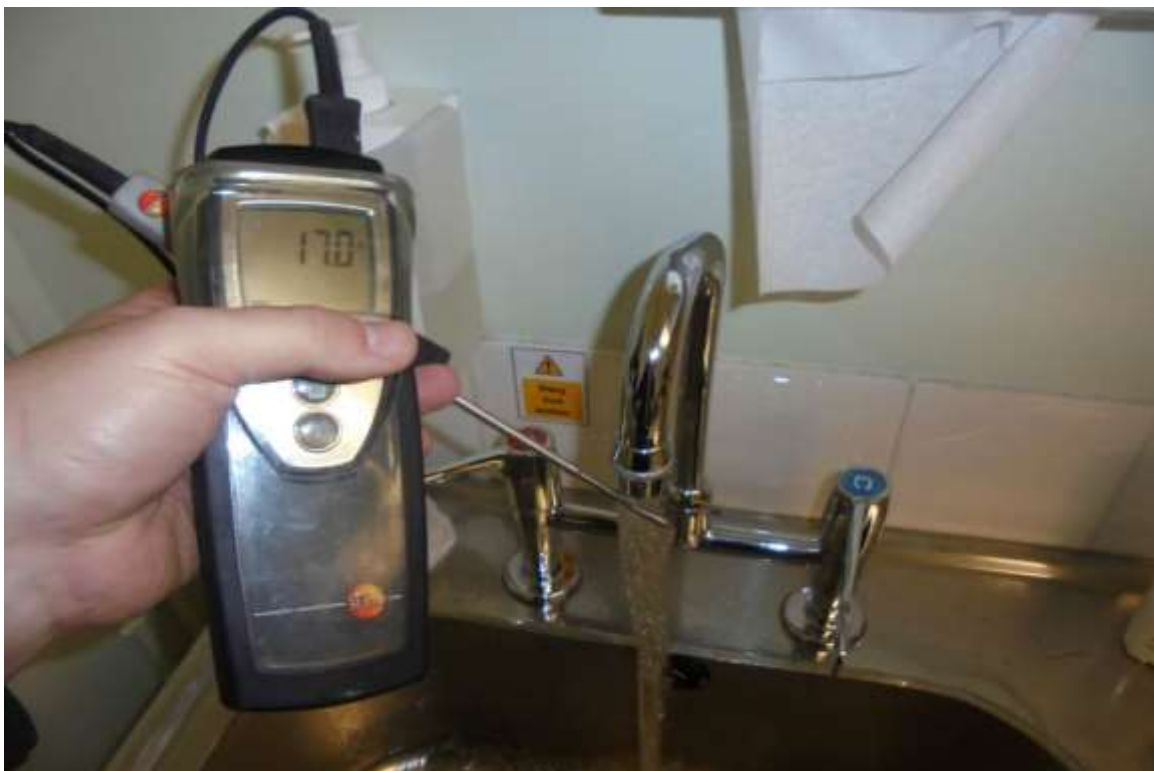
Treatment Room G/49 Sink – Cold Water Elevated After 2 Minutes
