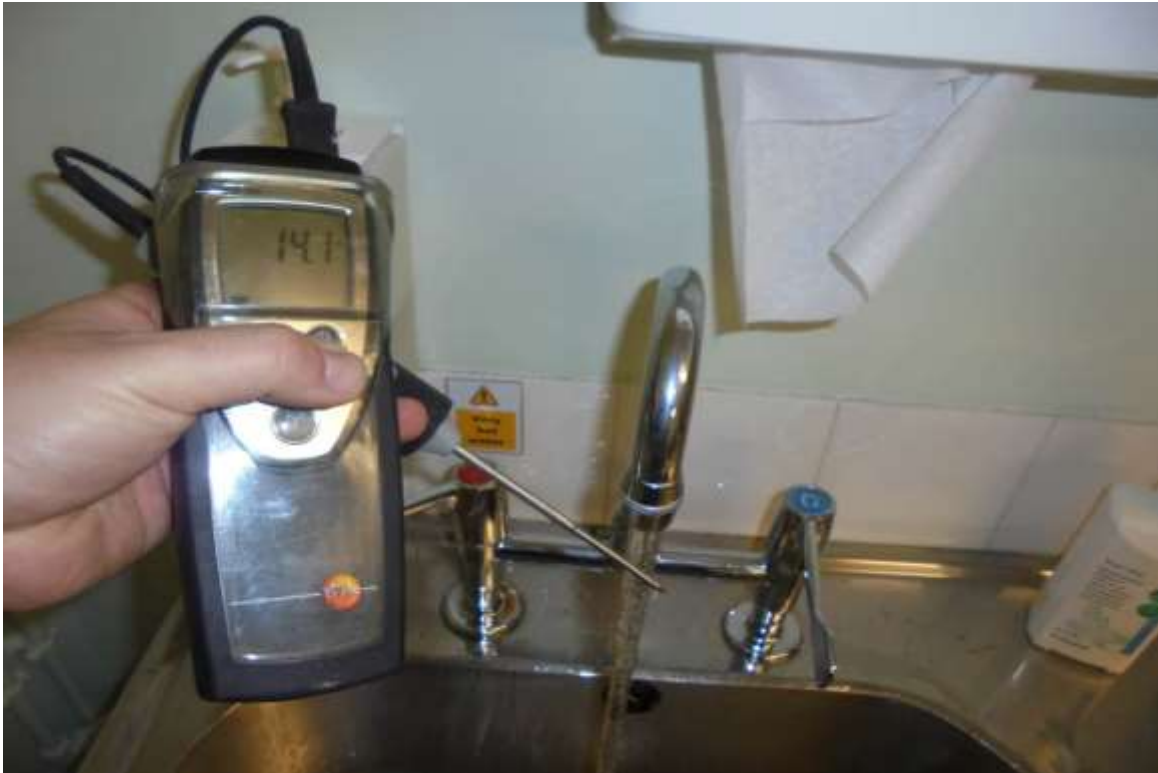
Treatment Room G/49 Sink – Cold Water Acceptable After Extended Flush
