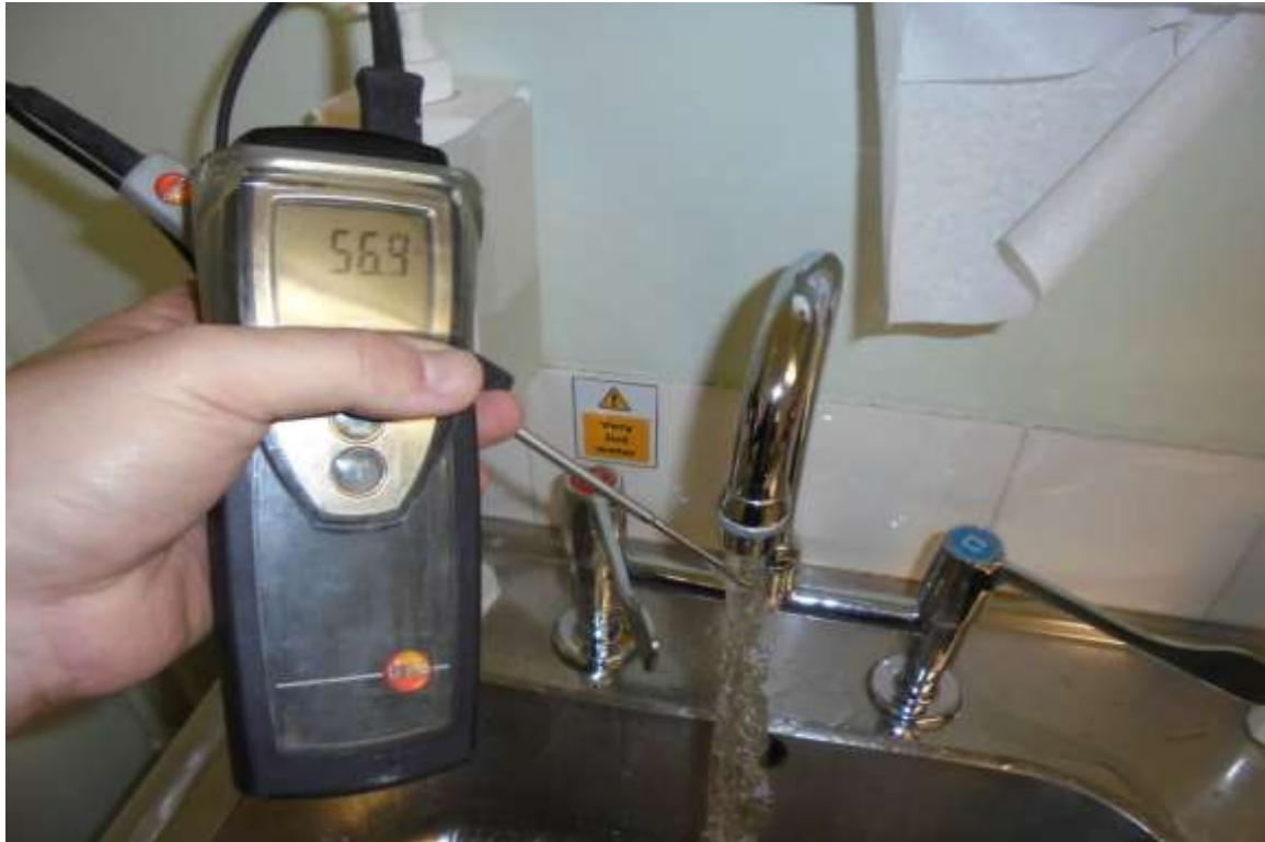
Treatment Room G/49 Sink – Hot Water Satisfactory After Extended Flush Ineffective Circulation
