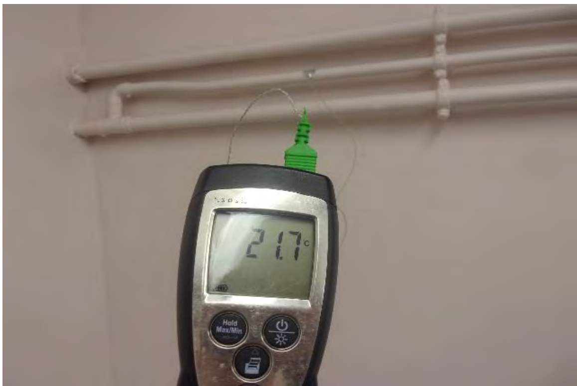
Store Room (G/34) Hot Water Return Temperature Too Low (<55°C)
