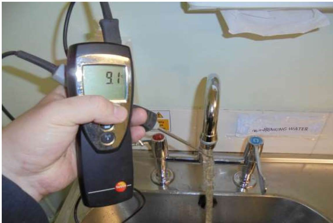
Consultant Room 8 Sink - Cold Water Outlet Temperature Satisfactory
