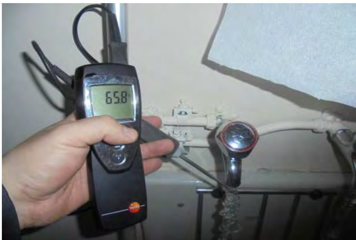
DSR Sink - Hot Water Outlet Temperature Satisfactory
