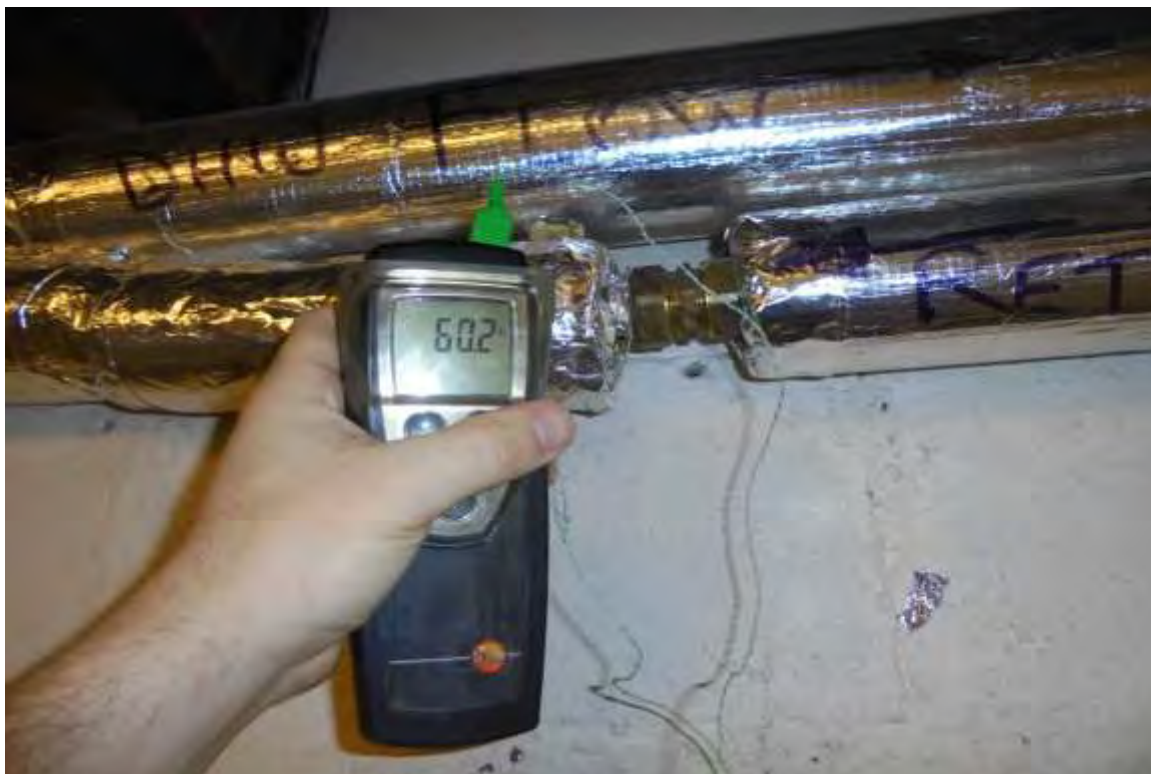
DHWS Return Temperature Satisfactory ( >55^{\circ}\text{C} )
