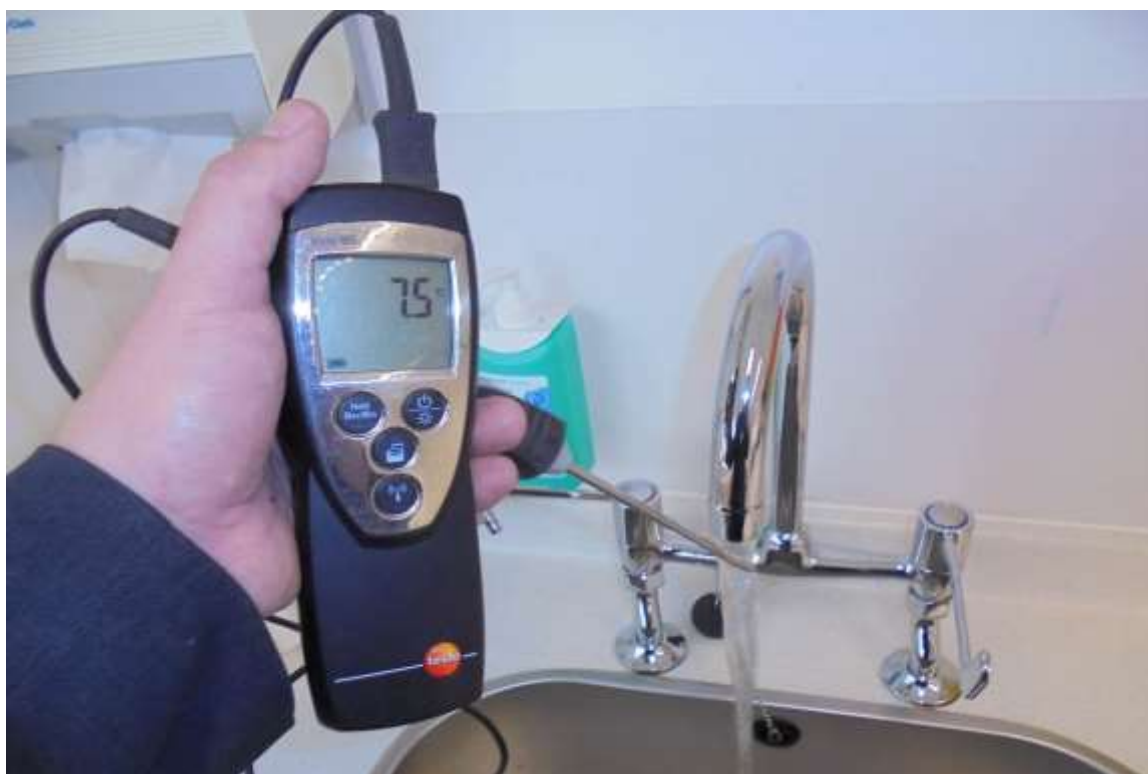
Extension Consultant Room 2 Sink - Cold Water Outlet Temperature Satisfactory
