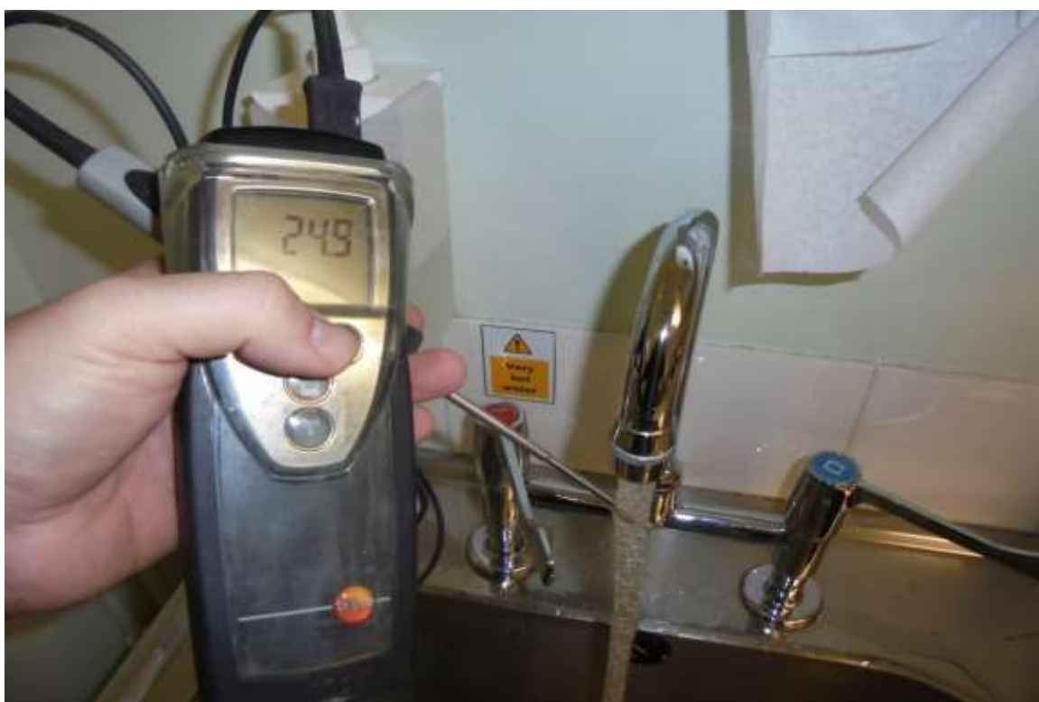
Treatment Room G/49 Sink – Hot Water Too Low After 1 Minute ( <55^{\circ}\text{C} )
