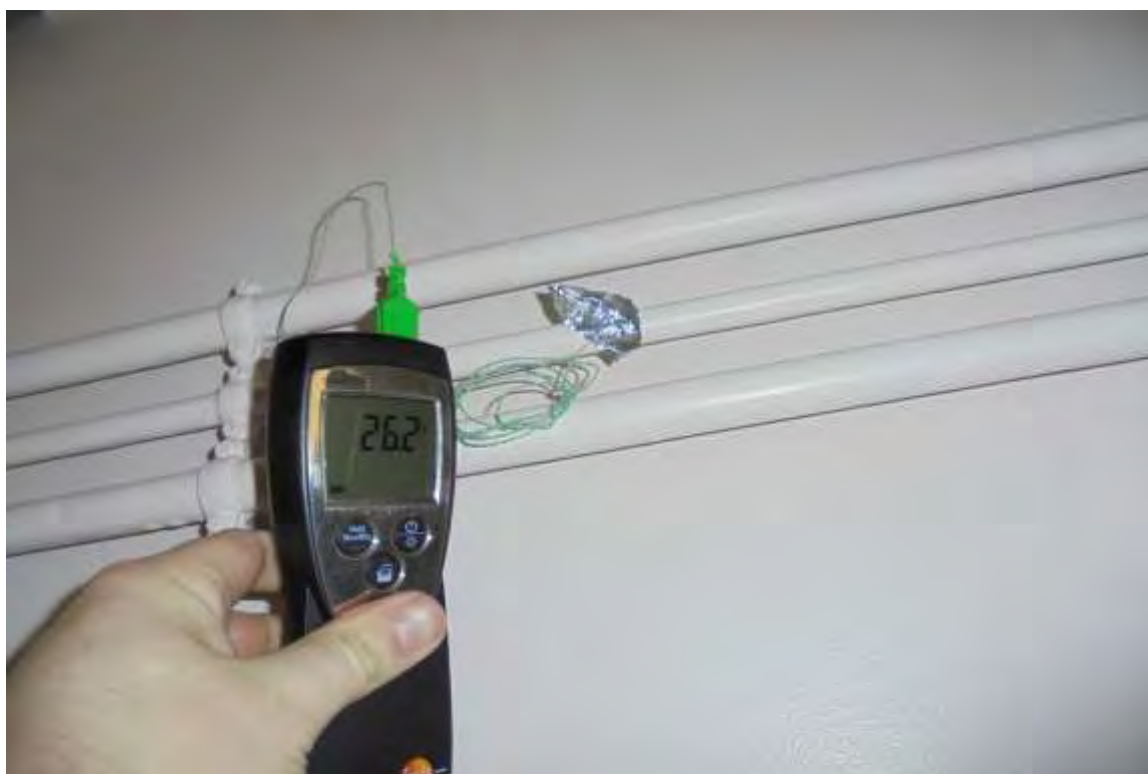
Health Education/Physio Room - Tertiary Loop Return Temperature Too Low (<55°C) After Flushing Outlet
