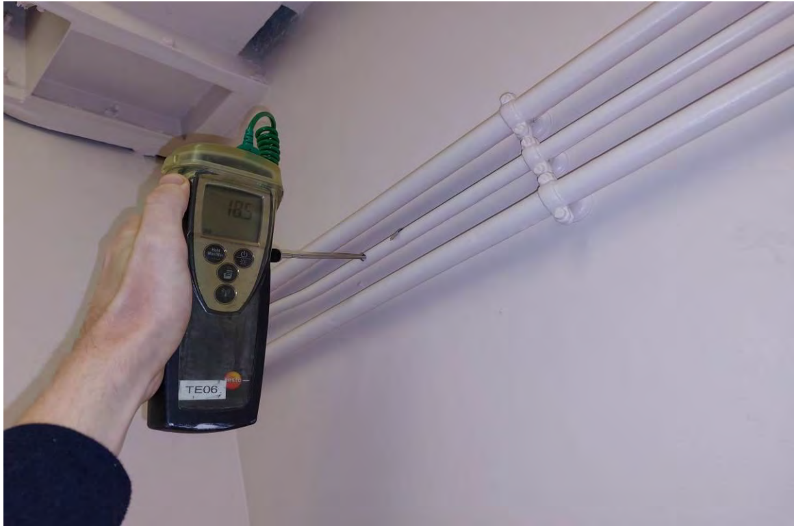
Health Education/Physio Room - Tertiary Loop Return Temperature Too Low (<55°C) Ineffective Circulation
