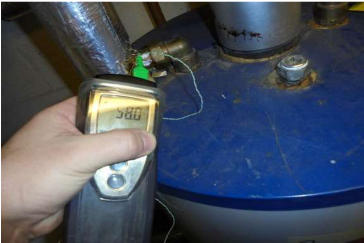
Gas Fired Water Heater No. 2 – Contents Temperature Confirmed at 58°C
