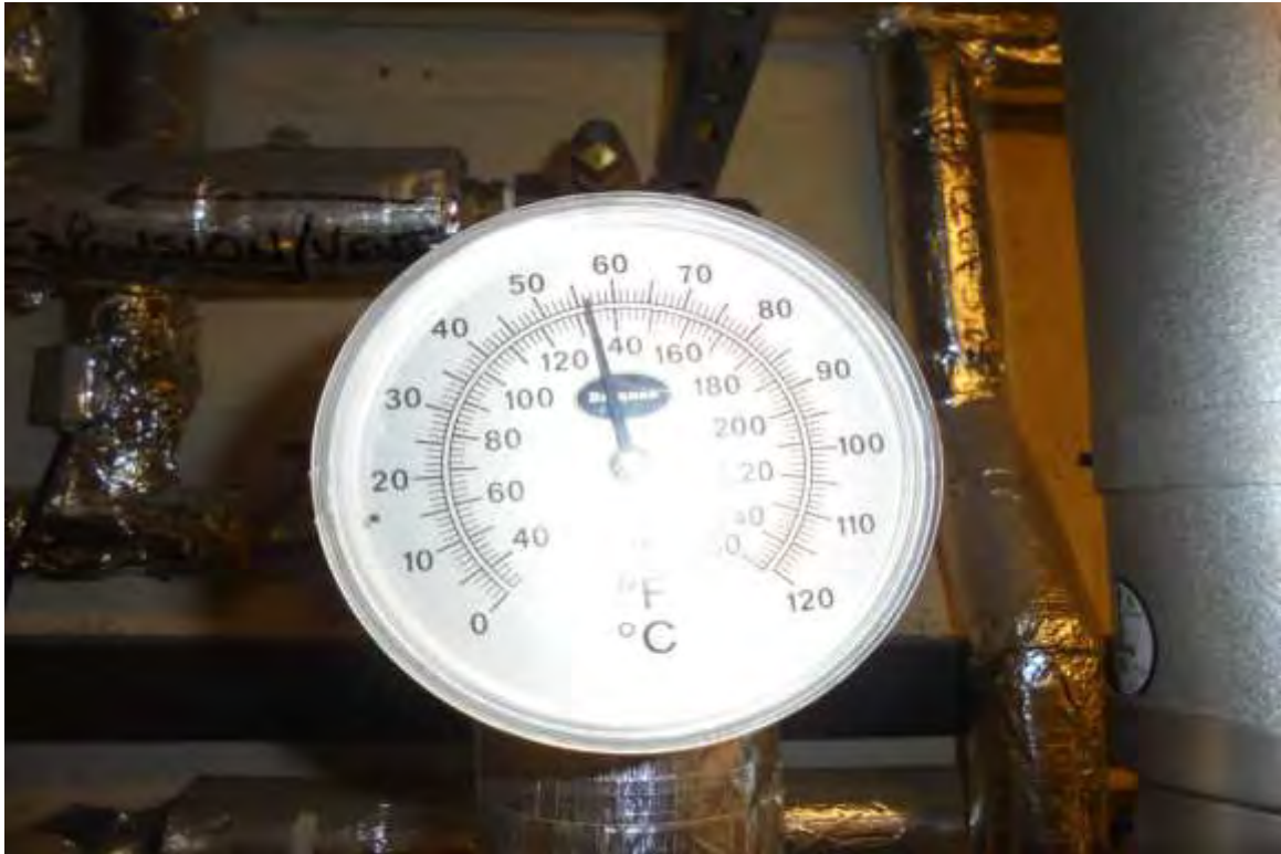
Gas Fired Water Heater No. 2 – Contents Gauge at 56°C
