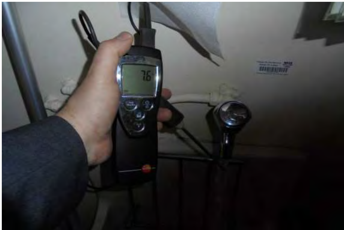
DSR Sink – Cold Water Outlet Temperature Satisfactory
