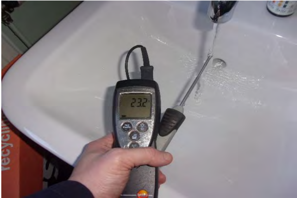
Secretarial Office (G/09) WHB – Cold Water Outlet Temperature Slightly Elevated (>20°C)
