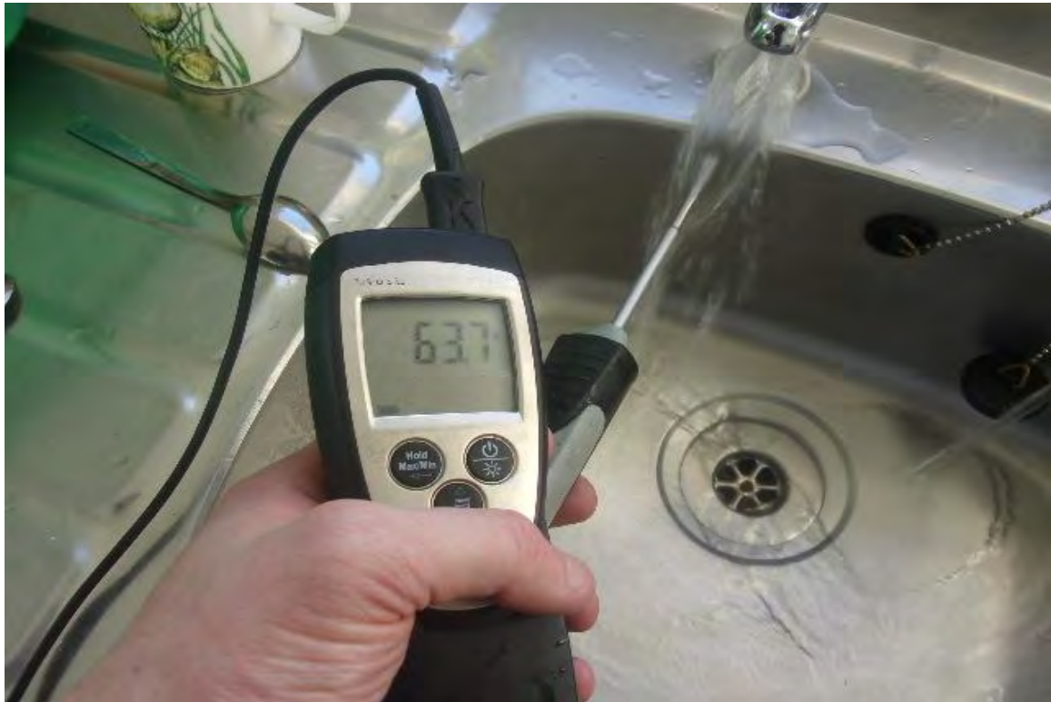
1 st Floor Staff Room Sink - Hot Water Outlet Temperature Satisfactory
