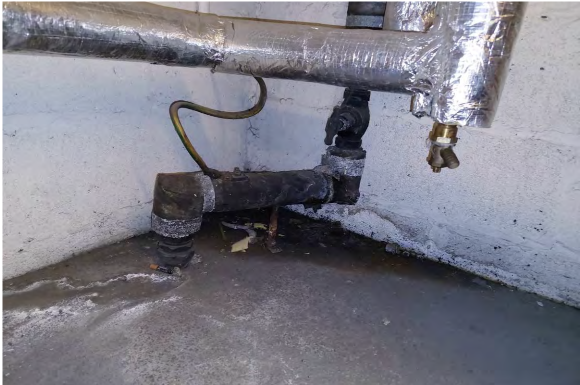
MWS Inlet with Stop Cock and Drain Point
