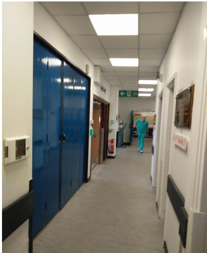
Figure 11 - Along the narrow theatre corridor, passing the main electrical switch cupboard, back to the lift on the stairwell
