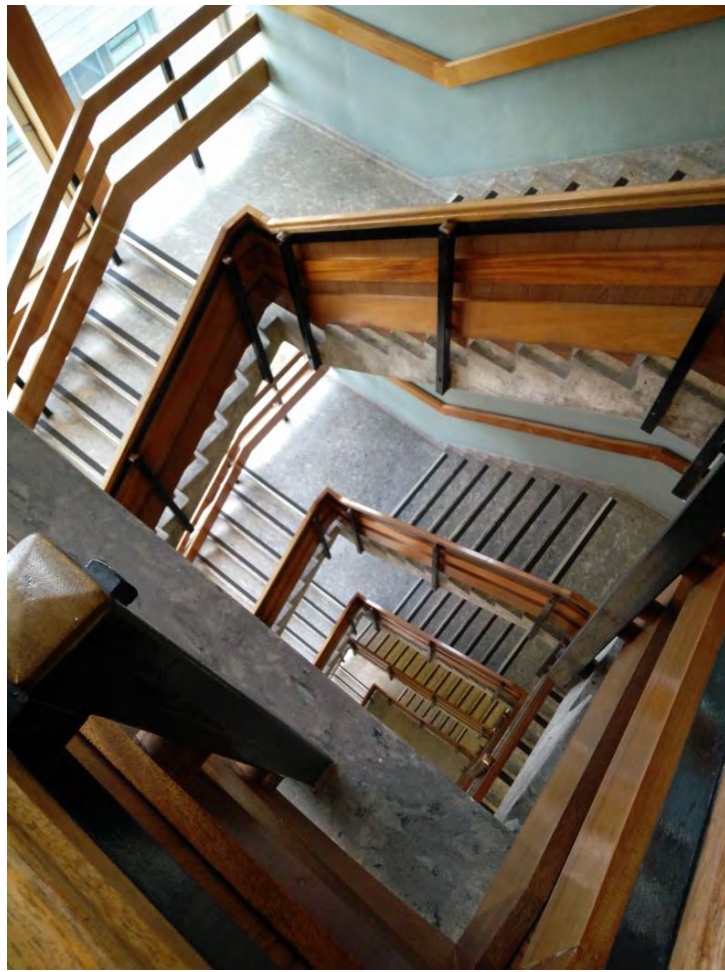
Figure 6 below: The main stairwell linking the 3 main outpatient floors, the ward, day bed suite, theatres and support accommodation. The alternative to the 2 lifts and the main evacuation route for patients and staff.
